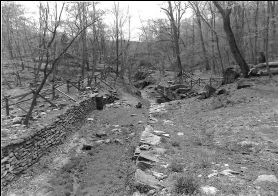
Photo 17 of 40 Canal segment between Locks 2 & 3 in the foreground, Lock 3 just visible beyond, view to SE (NR#43)
