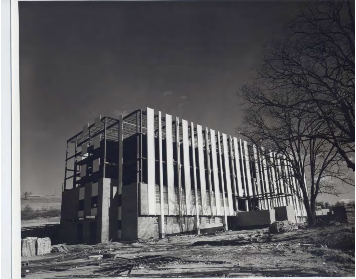
Figure 2. 1965 Photo of Smyth County Community Hospital Under Construction – Original South Façade and West Wall.
