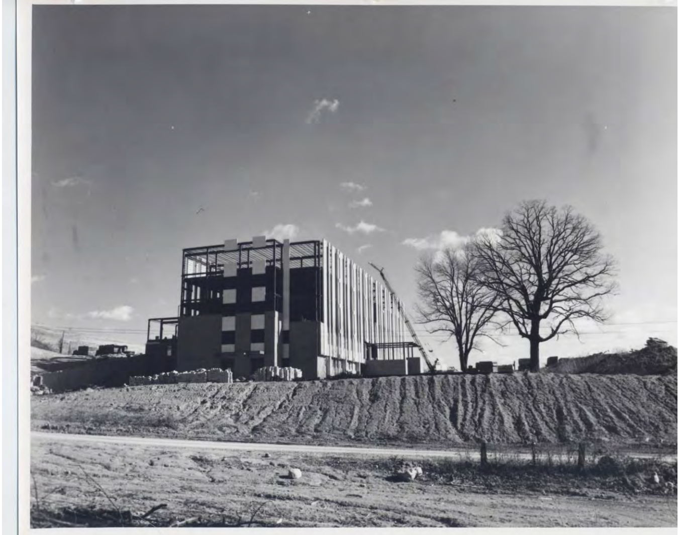
Figure 3. 1965 Photo of Smyth County Community Hospital Under Construction – Original South Façade at Right and West Wall at Left.
