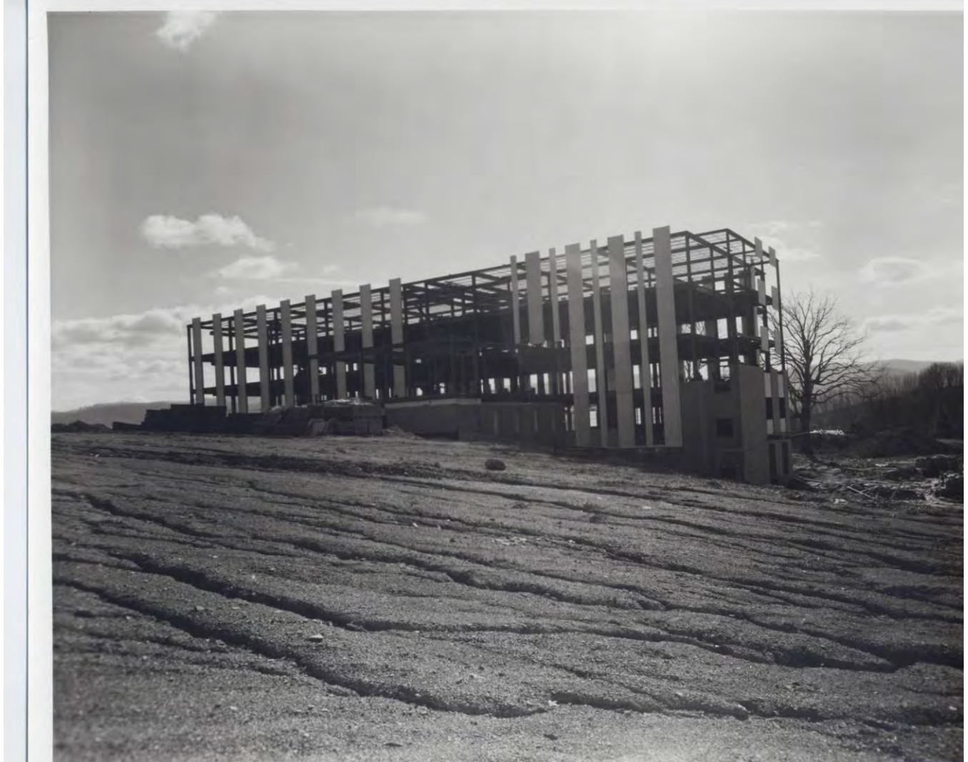
Figure 5. 1965 Photo of Smyth County Community Hospital Under Construction – Original North (Rear) Wall at Left and West Wall at Right.
