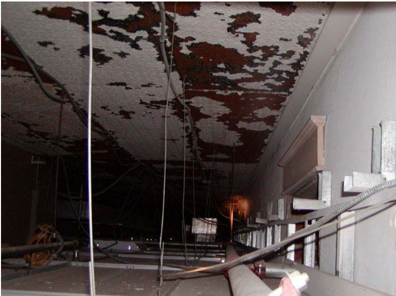
View above dropped ceiling tiles in corridor showing doors and transoms on right
