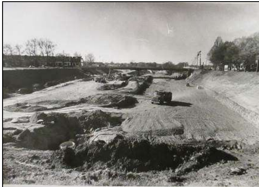
14. Construction of the Downtown Expressway, Looking West. Houses on the 500 block of S. Sheppard Street are visible in the left background and the Sheppard Street Bridge is at the center background. Source: The Valentine.
