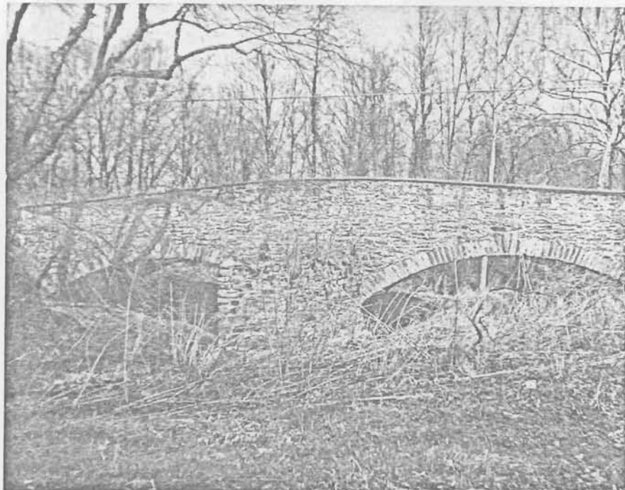
South side of the Little River Turnpike Companys stone bridge over the Little River, circa 1810. One of only two such structures remaining in use in all of Northern Virginia. Should be preserved at all costs. 53-244
