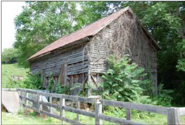
Figure 29: Lithia School #1 (011-5235). This ca. 1893 two-room school off Hardbarger Road in Lithia is currently used for storage and is in poor condition.
