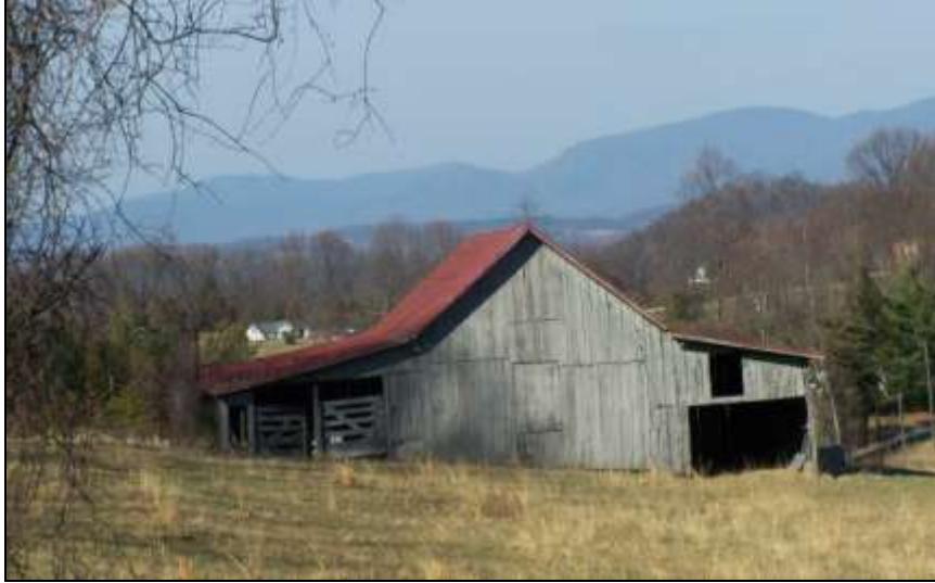
Figure 48: The large cattle barn, associated with the Max Brugh Farmstead (011-5202), is located in the adjacent field and is covered with vertical wood planks, the steeply pitched gable roof is covered with standing seam metal.
