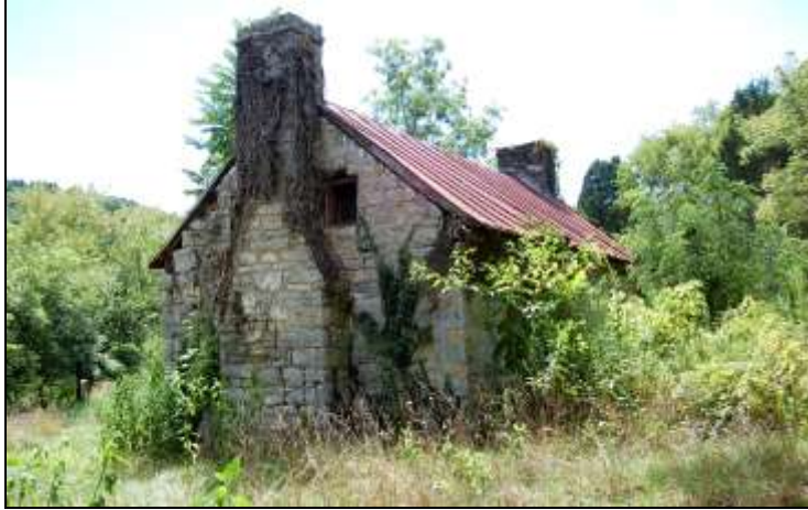
Figure 18: Pearl Alphin House (011-0138), present-day. The stone house now sits vacant and threatened by deterioration off of Route 622.
