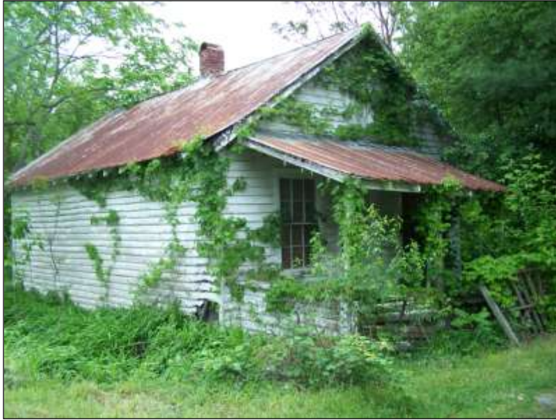
Figure 41: A good example of a rural country store is the ca. 1920 Store (011-5290) on Little Catawba Creek Road. It lies in an undeveloped area near the Craig County and Roanoke County lines. The one-story, three-bay frame building is currently vacant and threatened.
