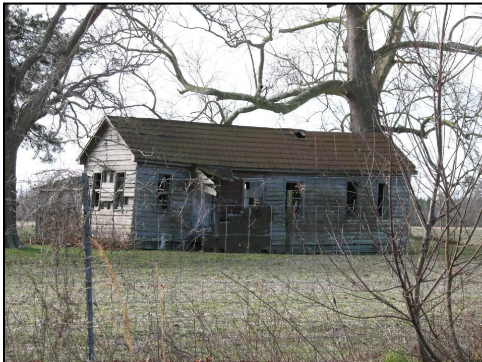
Figure 8. Tenant House located on the Property of 3116 Battlefield Boulevard (VDHR #131-0328), View Looking Southwest.
