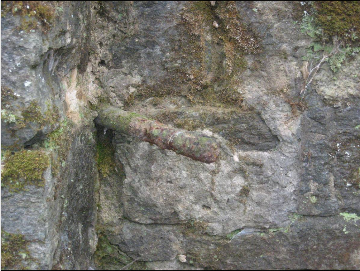
Photo 84: Metal Rod Protruding from Canal Lock 10 Foundation (44CU0034).
