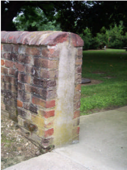
Above: Brick wall with modern patching.
