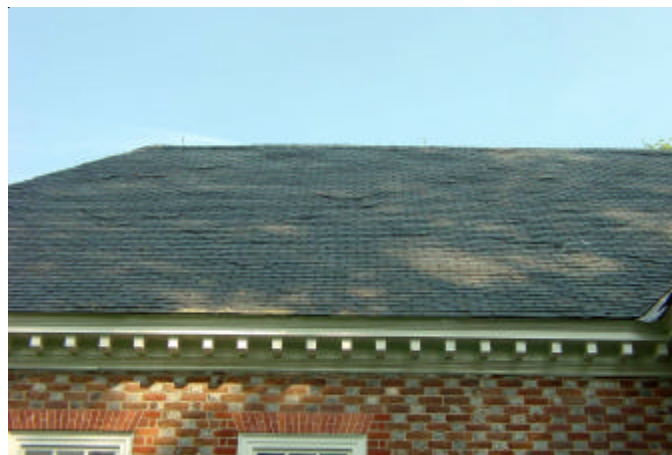
Above: In raking light many patches of roof shingles can be easily discerned because the later shingles do not match the thickness of the earlier shingles.
