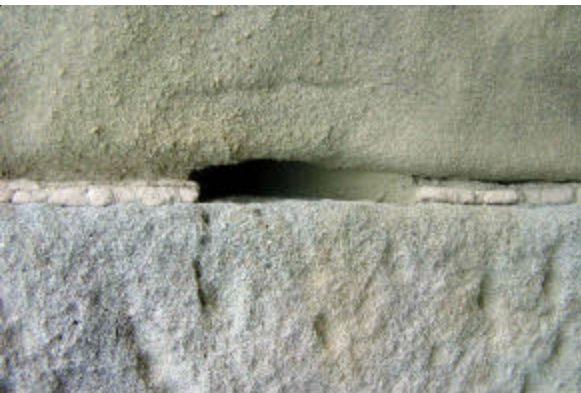
Above: Many mortar joints have completely deteriorated and require re-pointing.
