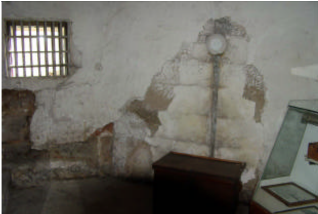
Left: This firebox in the northeast cell should once again be opened to allow air to circulate within the chimney flue.
