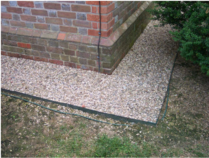
Above: Foundation drainage system.
