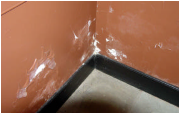
Above: Rising dampness is destroying the plaster in the north and south wings.
