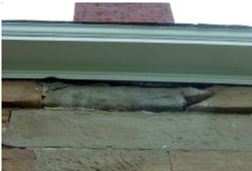
Above: The stone beneath the chimney deteriorated when water was allowed to flow around the flashings of the chimney. This leak does not appear to be active.
