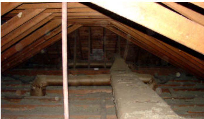
Above Left: Both fireplaces in the north and south jury rooms have been sealed. These should be opened to allow the flues to ventilate.
