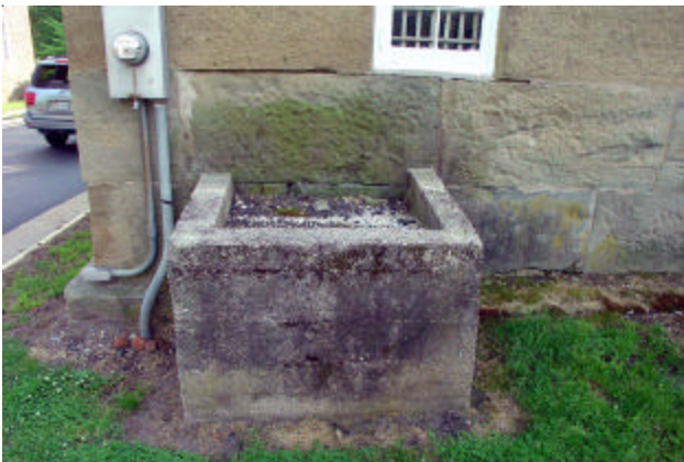
Above: This is one of two cesspits that once served the cells within. These are now keeping water against the original stone walls and causing deterioration.
