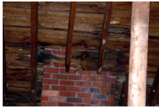
Above: A close view of the roof deck deterioration around the chimney within the attic.
