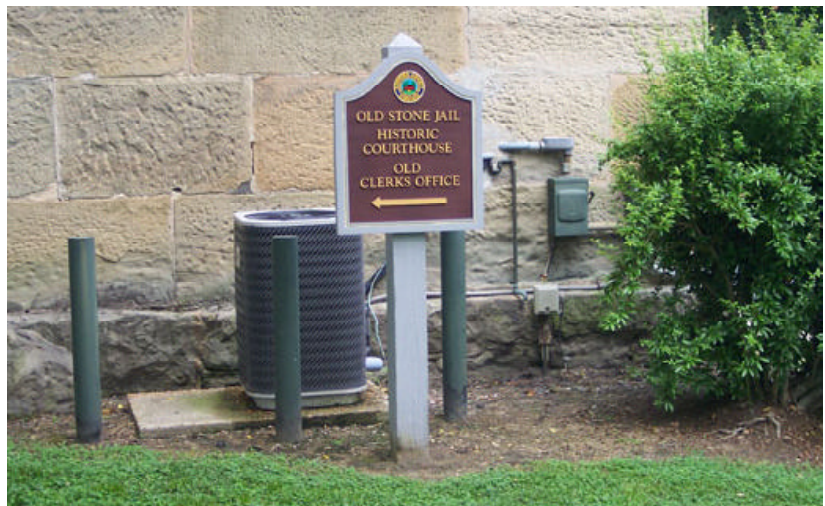
Above: Electrical devices and panels mounted on stone wall of jail.
