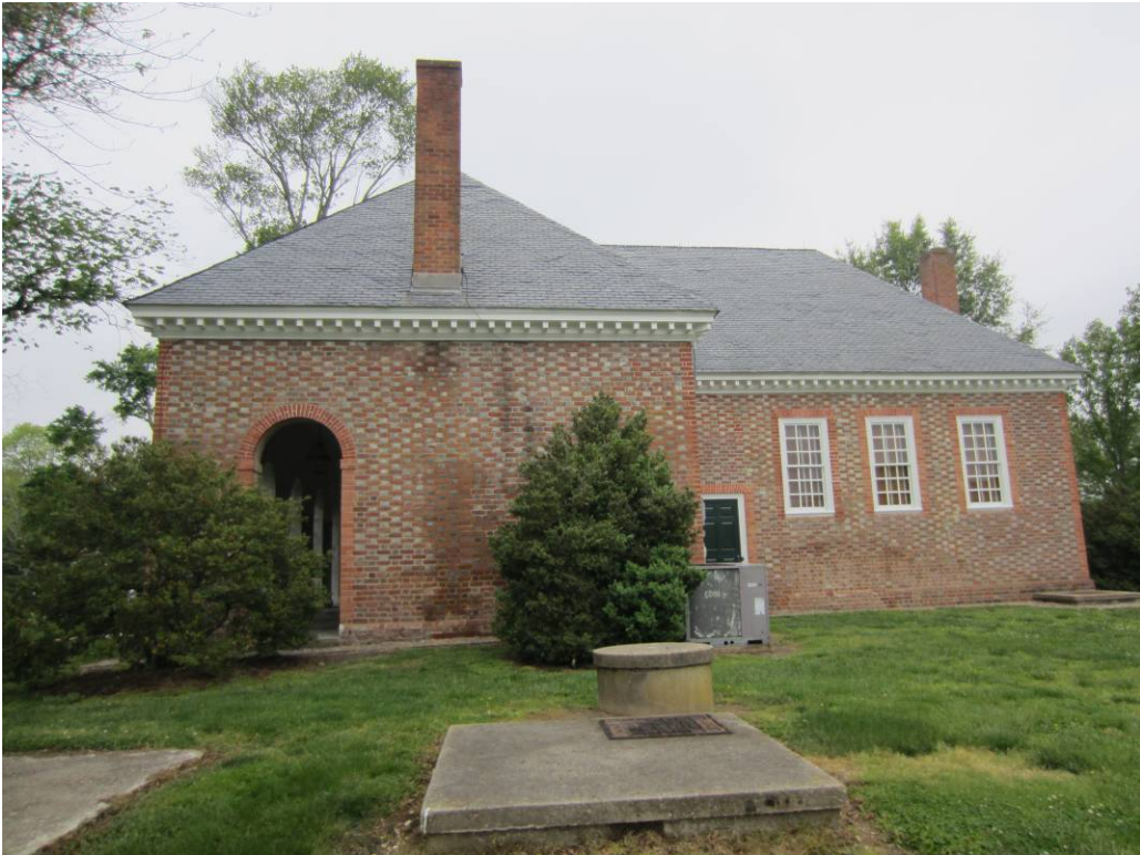
The south elevation after treatment (darker areas visible on the masonry walls are due to moisture from early morning rainfall).
