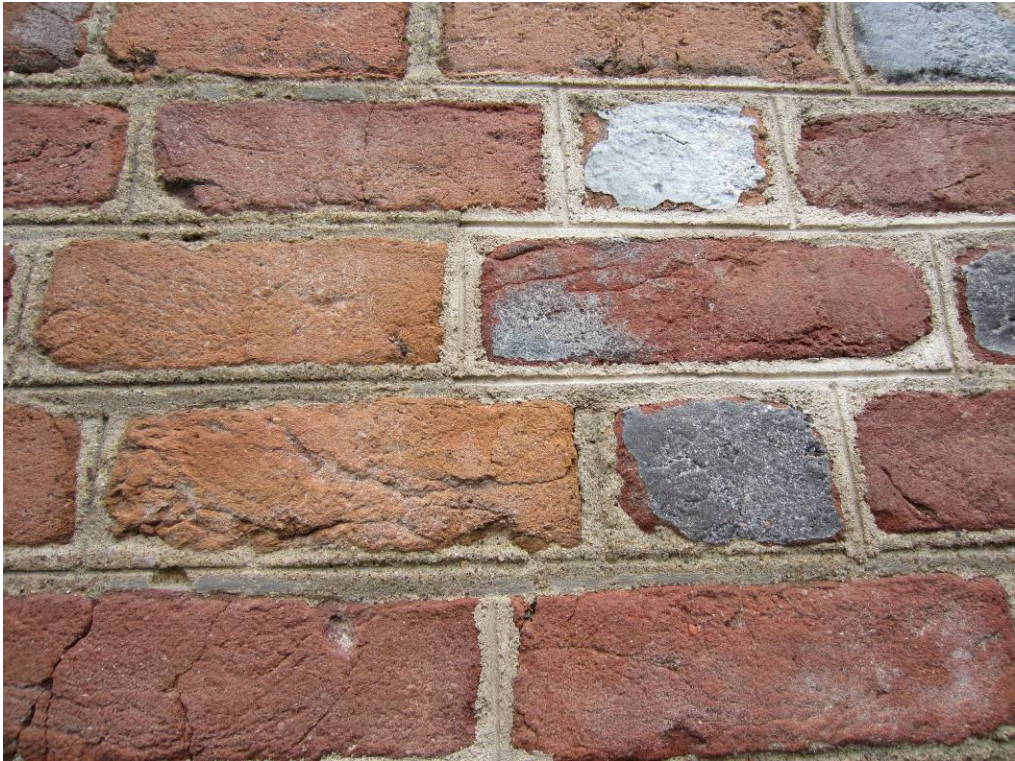
Close-up of new repointing work next to historic repointing work on the south elevation.
