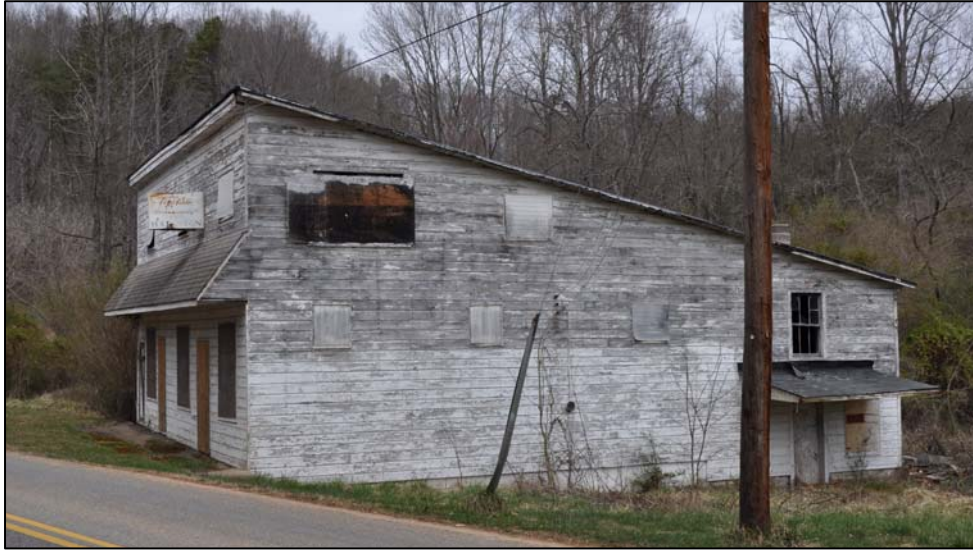
Figure 42: The important ca. 1920 Early Hairston Store (044-5277) that fronts Mary Hunter Drive just south of Bassett in an African-American hamlet that Early Hairston established. The hamlet includes his house along with a dozen or so workers' houses where the residents trekked over the hill that separated them from Bassett and the factories where they labored.
