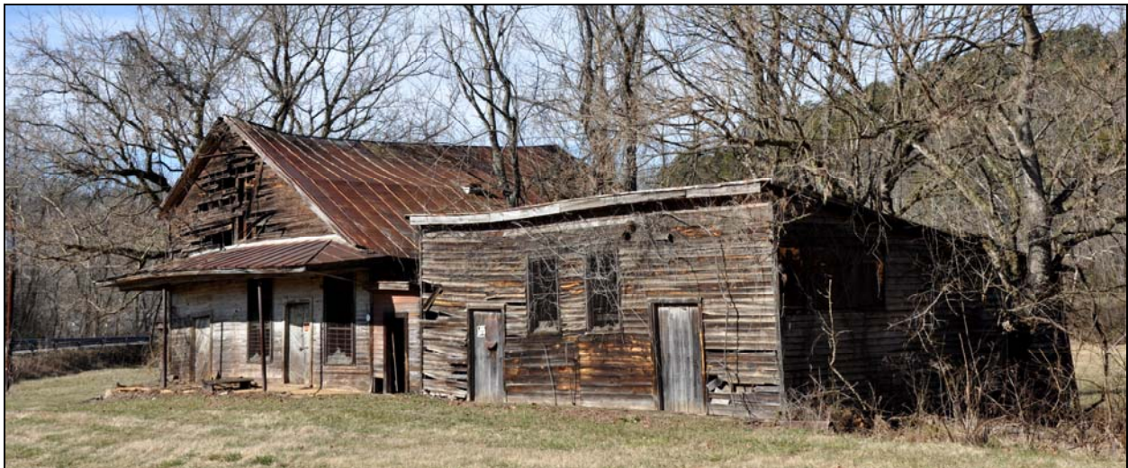
Figure 20: The 1905 Philpott Mercantile Store (044-5222) is a rare example of an early twentieth-century commercial building that served the community of Philpott along the Smith River. The building is vacant and threatened.
