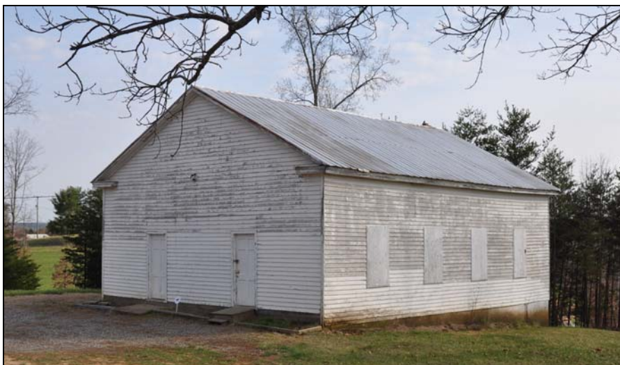
Figure 23: The ca. 1875 Leatherwood Church (044-5284) provided two separate entrances that segregated the sexes of the congregation. The plain structure features a return cornice and rests on a fieldstone foundation.
