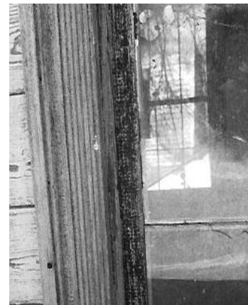
Figure 57: Window detail at the Jeter House (055-5036)
