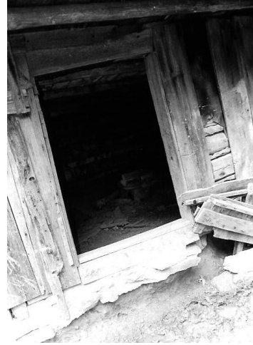
Figure 73: Interior of Sweet Potato House showing clay burner, ca. 1840, White Oaks Farm (055-5072)
