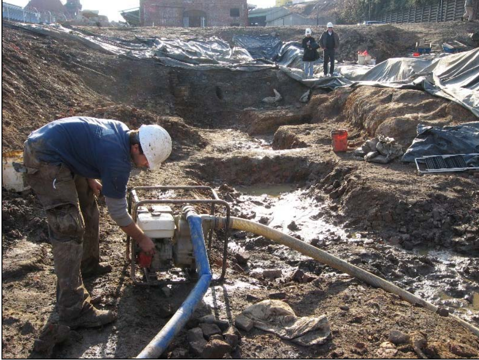
Figure 83. Dewatering the lowest part of the site near the jail building foundation.
