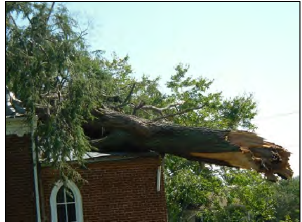
Figure 44- Christ Church (062-0003) was damaged by a September 2012 storm (photo courtesy: J.P. Harvey, nelsoncountylife.com)
