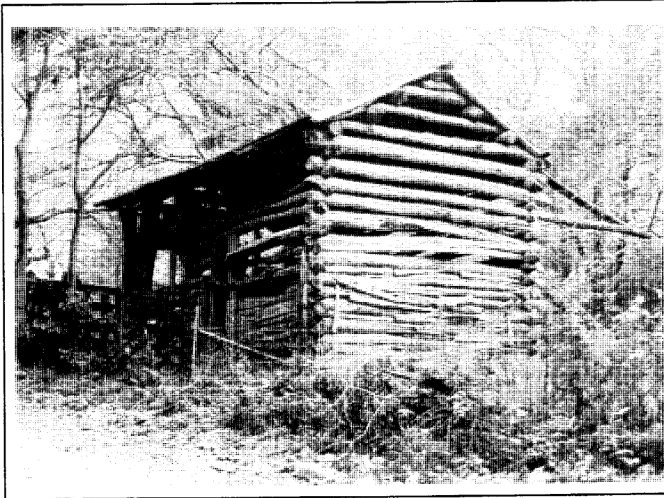
Fig. 14. This single-crib log barn at the head of Jollett's Hollow (069-5028) may be typical of the small-scale barns that once populated Page County's less prosperous upland farms. A notable feature is the barn's log purlin roof, a construction form that was common during the early years of Page County's settlement but rare by the end of the nineteenth century as nail availability and sawmill technology made nailed rafter roofs universal in small-scale construction. The barn probably dates to the first third of the twentieth century, so its roof represents a holdover of an archaic form.
