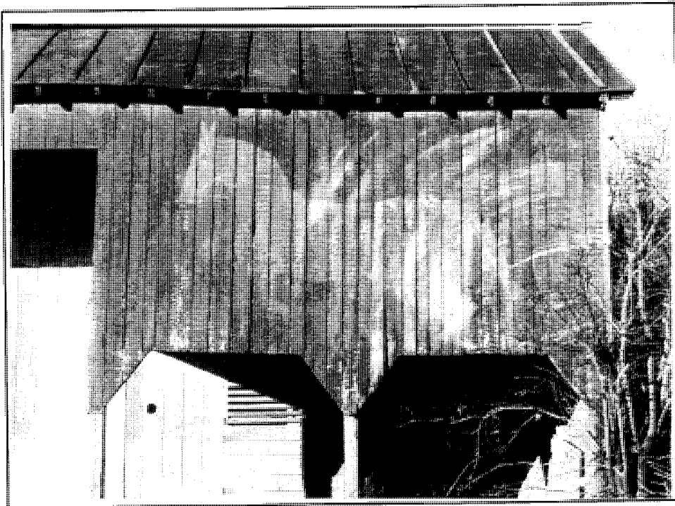
Fig. 49. The Griffiths Barn (069-5050), built in 1917 in the Morning Star vicinity, preserves traces of farm-scene painting executed by Luray house painter Vernon Housdon.
