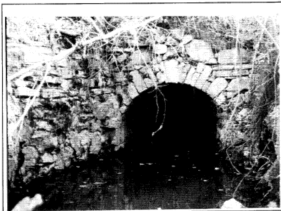
Fig. 16. Sandy Hook Mills (069-5001), located at the confluence of Hawksbill Creek and the Shenandoah River, was probably established in the 1700s. The mill is in ruins, but an unusual underground mill race survives. The race channeled water under a ridge that protected the mill building itself from flooding on Hawksbill Creek.
