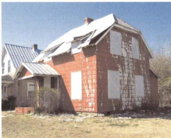
The boarded-up windows on this vacant house display the original pattern of window placement.
