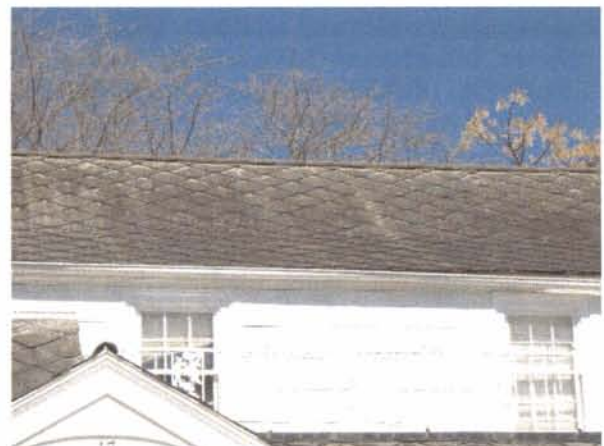
The original roofing material can still be found on a number of dwellings in the district.
