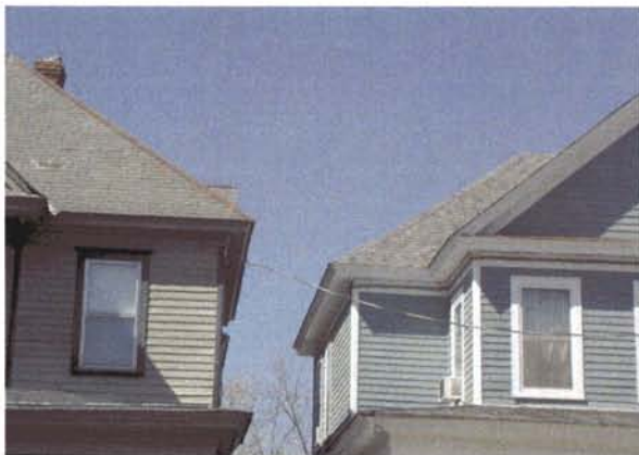
The original slate roof (left) has been replaced by architectural shingles (right).
