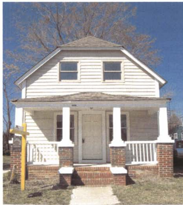
Inappropriately sized replacement windows change the appearance of this example.
