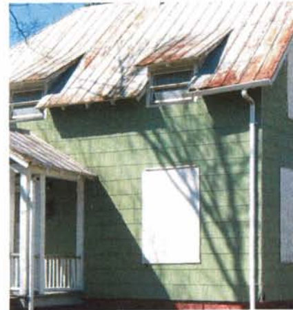
The original wood siding on this vacant house was covered with asbestos shingles which appear to be in good condition.
