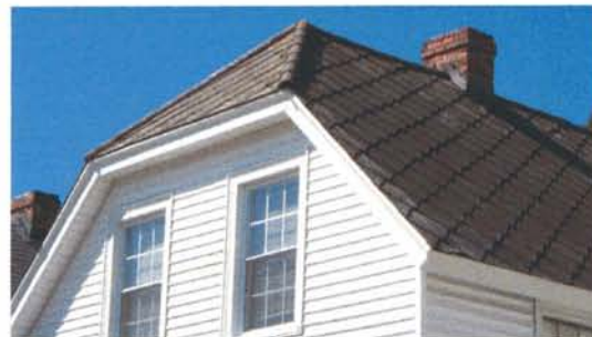
Diamond-shaped asbestos-cement shingles were the original roof material in Truxtun.
