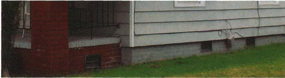
These foundation vents are free from vegetation that could block the circulation of air under the house.
