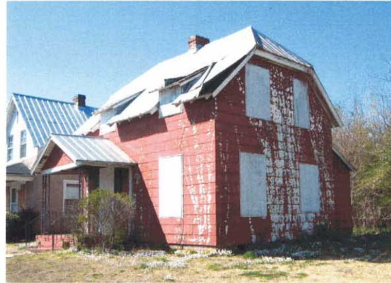
Even vacant structures need to be maintained to prevent deterioration of the structure until a rehabilitation can be undertaken.
