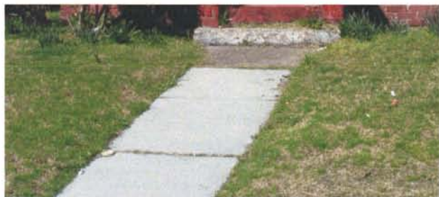
A resurfaced or repaired walkway shown here illustrates the contrast between the warm tones and rough texture of the old concrete and the new gray smooth concrete lacking aggregate.
