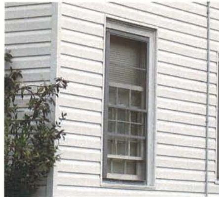
By lowering the upper sash, a homeowner can allow warm air to exit. Raising the lower sash allows cooler air to enter the house.
