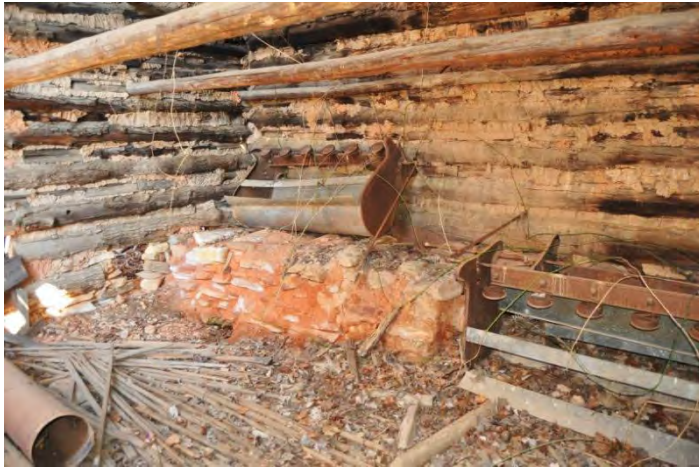
An oil burner next to an intact stone firebox.
