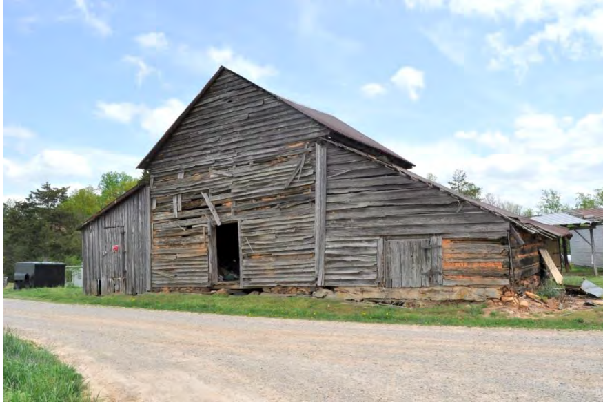
A pack barn owned by the Sparks Family in Pittsylvania County is partially log-constructed and partially wood-framed.
