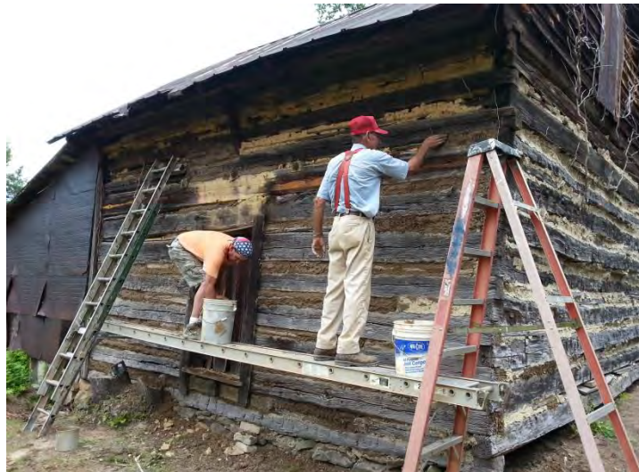
M and M Construction repairing a tobacco pack barn as part of Preservation Virginia/JTI Mini-Grants Project to repair barns in a 3-county region.
