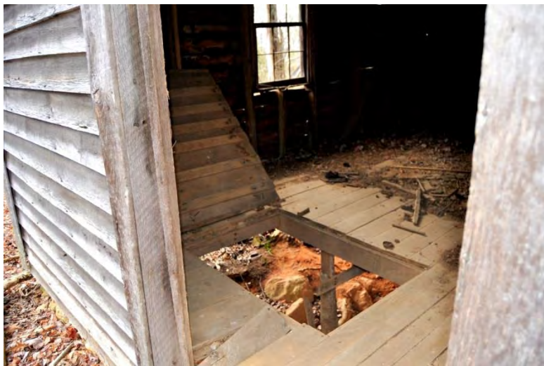
View of a severely eroded ordering pit in a pack barn. Interior trap doors usually lead to the ordering pits.
