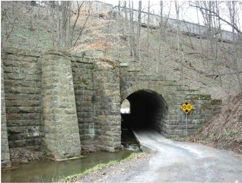
Figure 195. Buttressed and stepped wing-walls, Thompson Creek Tunnel #1 (083-5016), Thompson Creek Road, near Honaker (2008).
