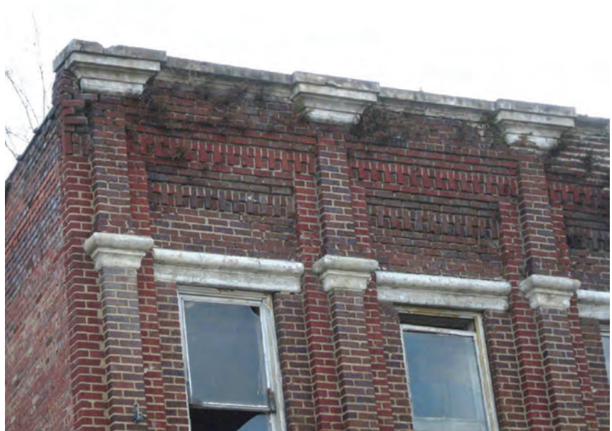
Figure 42. Cornice details, Ball's Cash Store (239-5003), Tunnel Hill Road, Honaker (2008).
