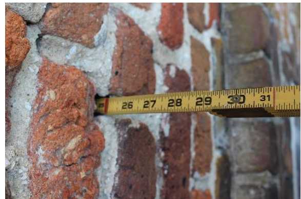
Figure 5.7, Bacon's Castle, South elevation ca. 1665 building, extreme mortar loss. In this instance, the carpenter's rule was inserted through the entire wall (approx. 18" thick at this location), and was visible from the interior of the castle.
