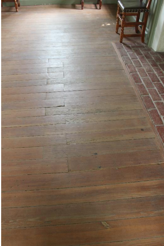
Figure 5.144, Bacon's Castle, ca. 1665 building, West Room, Room 103, detail of floor. Note the sawn and replacement floorboards.
