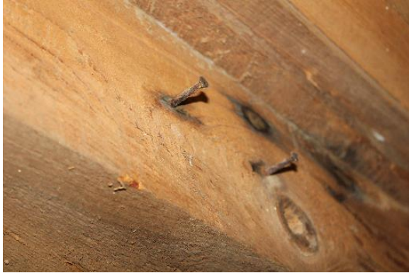
Figure 5.90, Bacon's Castle, ca. 1665 dwelling, Basement, West room, Room 005, summer beam. Note the nails, which were used in the construction of the plank wall that previously divided the room.
