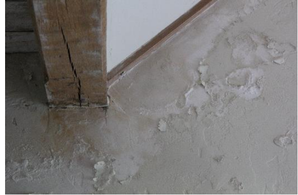
Figure 5.67, Bacon's Castle, ca. 1665 dwelling, Basement, Room 001, crack in beam. Note the efflorescence.
