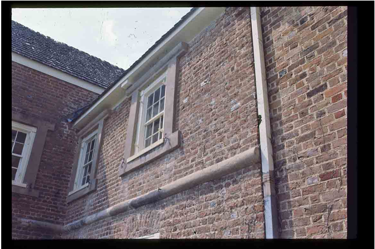
Figure 106: Bacon's Castle, detail view of east end of south façade, second floor, 1975. Courtesy Virginia Department of Historic Resources.
