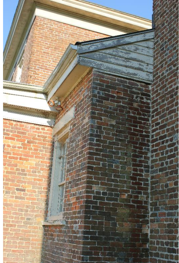
Figure 5.53, Bacon's Castle, West elevation, Hyphen cornice detail, ca. 1950s kitchen addition cornice detail, ca. 1854 addition cornice detail.
