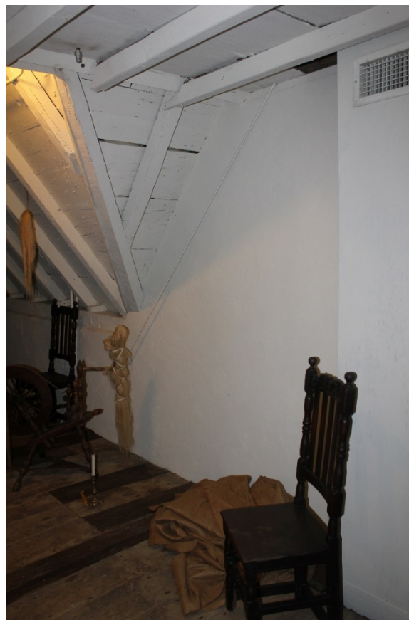
Figure 5.245, Bacon's Castle, ca. 1665 portion, Garret Floor, Room 303, detail of modern ductwork.
