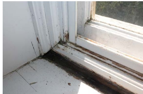
Figure 5.202, Bacon's Castle, ca. 1665 building, Second Floor, South Tower, Room 204, detail of water infiltration and rotting sill.
