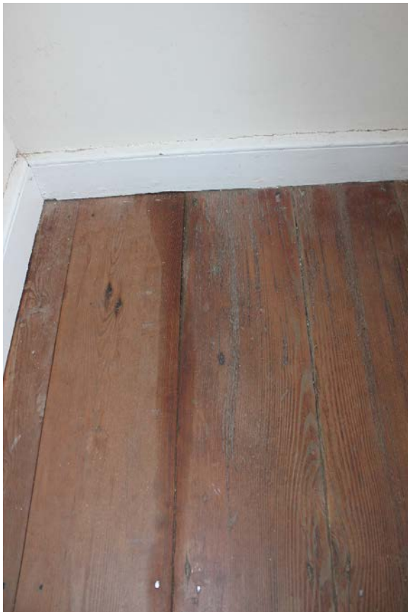
Figure 5.192, Bacon's Castle, ca. 1665 building, North Tower, Second Floor, Room 201, detail of floorboards showing water damage.
