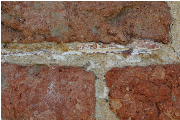
Figure 2.12: Bacon's Castle, South elevation (primary), immediately under eaves. Note surviving red lime wash on joints with white penciled joints on top. Photograph 26 July 2015.
