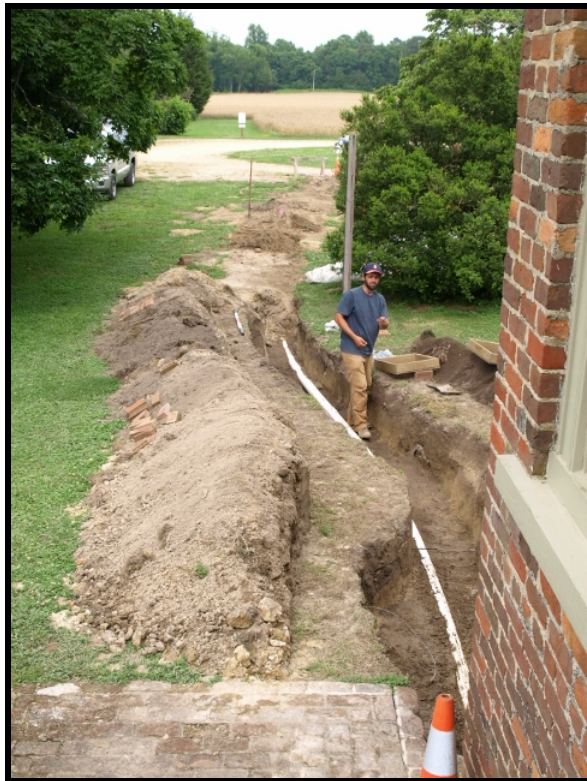
Figure 3.21: Replacement septic line trench extending off the northeast corner of the 1854 wing, ER800.
