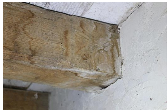
Figure 5.68, Bacon's Castle, ca. 1665 dwelling, Basement, Room 001, Note the water marks on the beam.
