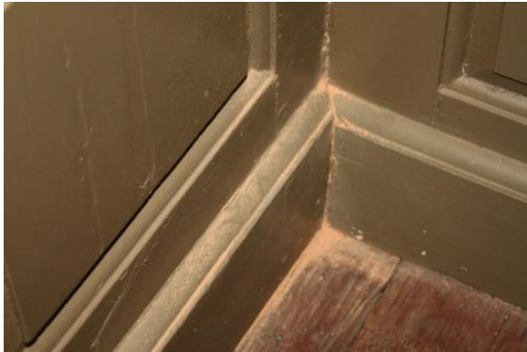
Figure 5.155, Bacon's Castle, ca. 1665 building, East Room, Room 105, brick and mortar dust seeping through the walls.
