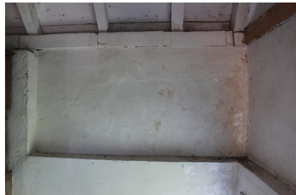
Figure 5.232, Bacon's Castle, ca. 1665 portion, Garret Floor, Room 301, detail of west wall. Note how the wall thickness changed. Note the efflorescence.
