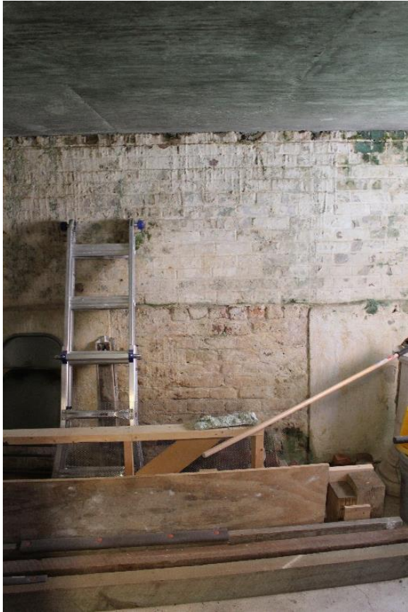
Figure 5.118, Bacon's Castle, Basement, Room 011, storage space. Note biological growth.
