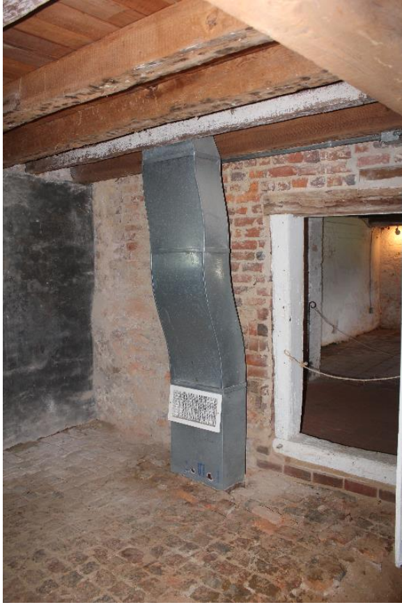
Figure 5.94, Bacon's Castle, ca. 1665 dwelling, Basement, West room, Room 005, ductwork.
