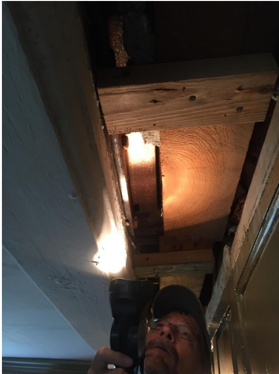
Figure 2.88: Bacon's Castle, first floor, east room (Hall). Material has been removed in vicinity of ceiling plaster crack and beam crack to reveal steel reinforcement. 31 July 2015. Commonwealth Architects
