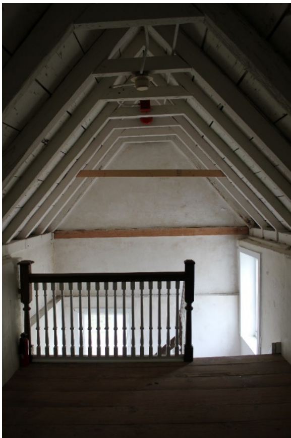
Figure 2.135: Bacon's Castle, Garret, stair tower (north) view to north. Photograph Commonwealth Architects, 2015.
