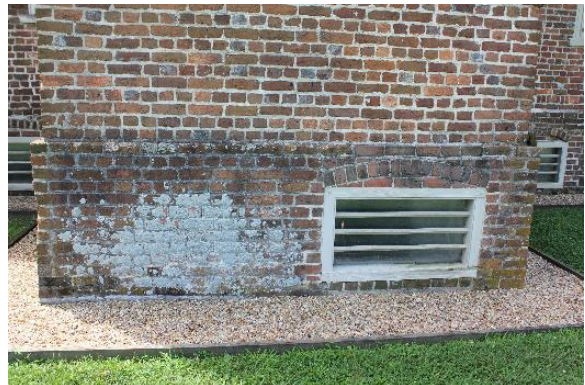
Figure 5.29, Bacon's Castle, North elevation, detail of foundation. Note the biological growth.
