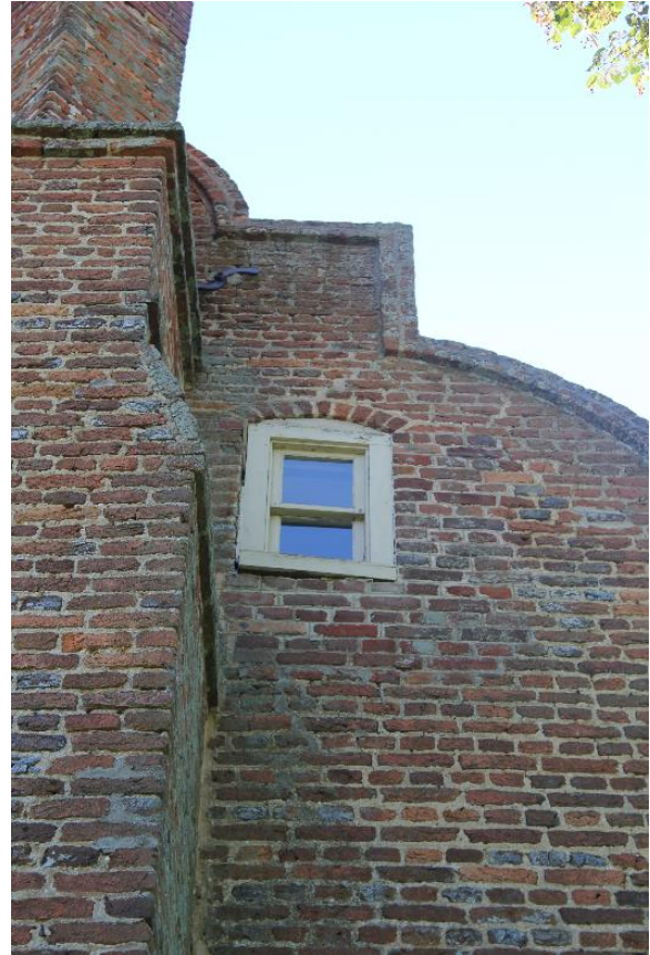
Figure 5.56, Bacon's Castle, West elevation, garret level window. Note how the fireplace mass is warping the west wall of the castle. The window is also being pulled with the wall.
