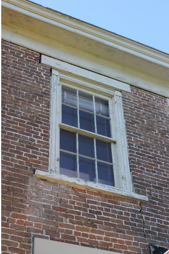
Figure 5.23, Bacon's Castle, North elevation, detail of ca. 1854 addition second floor window. Note the sheared bricks beneath the lower right corner of the window and the separation of the wall from the window frame on the left side of the window. Efflorescence is also present beneath the lower left corner of the window.
