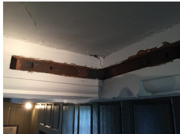
Figure 2.87: Bacon’s Castle, first floor, east room (Hall). Material has been removed in vicinity of ceiling plaster crack and beam crack to reveal steel
