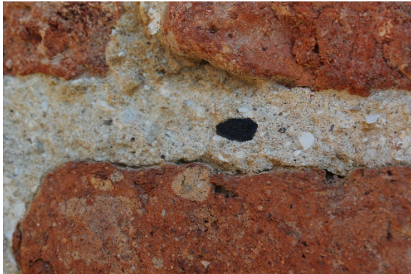
Figure 2.11: Bacon's Castle, South elevation (primary), immediately under eaves. Note irregular mortar joints, uneven brick margins, large aggregate. Photograph 26 July 2015.
