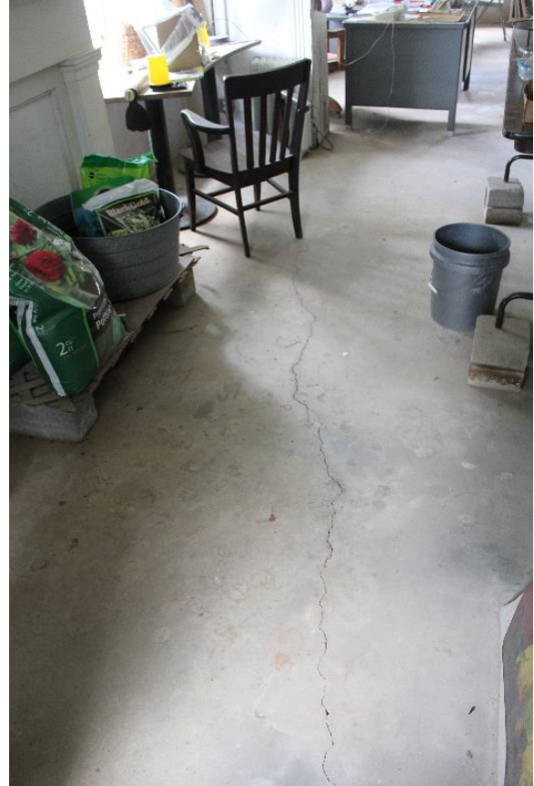
Figure 5.110, Bacon's Castle, ca. 1854 addition, Basement, Room 008,009, concrete floor. Note the large crack. Also note the gardening supplies. They have been elevated above the floor with concrete masonry units and a board.
