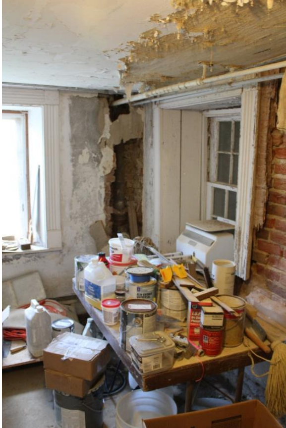
Figure 5.102, Bacon's Castle, ca. 1854 addition, Basement, Room 007, Window details. Note demolished portion of southwest corner, missing portion of window trim, and plaster ceiling damage.
