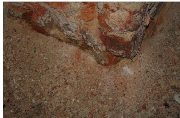
Figure 5.124, Bacon's Castle, Hyphen, Room 012, pile of brick and mortar dust.
