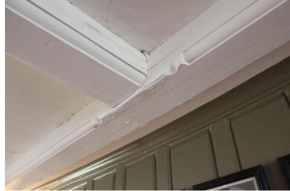
Figure 5.151, Bacon's Castle, ca. 1665 building, East Room, Room 105, beam detail above fireplace. Note the cracking.
