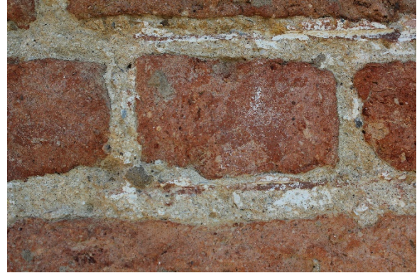
Figure 2.13: Bacon's Castle, South elevation (primary), immediately under eaves. Note surviving red lime wash on joints with white penciled joints on top. Photograph 26 July 2015.
