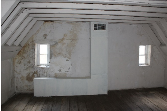
Figure 5.246, Bacon's Castle, ca. 1665 portion, Garret Floor, Room 304, view east. Note the extreme efflorescence and damaged plaster in the northeast corner.
