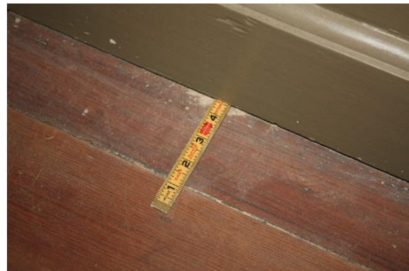
Figure 5.152, Bacon's Castle, ca. 1665 building, East Room, Room 105, carpenter's rule inserted through the entire depth of the exterior brick wall.
