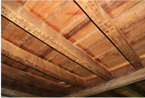
Figure 5.195, Bacon's Castle, ca. 1665 building, Second Floor, West Chamber, Room 203, ceiling detail. Note the nail marks from previous lath.
