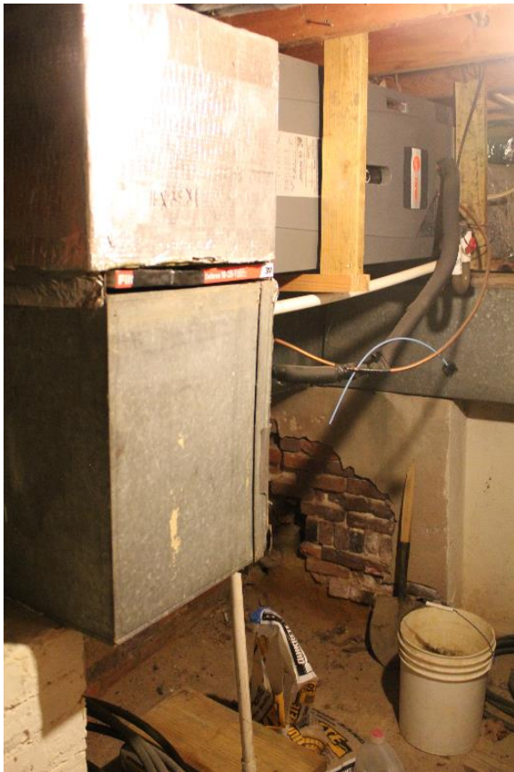
Figure 5.117, Bacon's Castle, ca. 1950s addition, Basement, Room 010, mechanical equipment.
