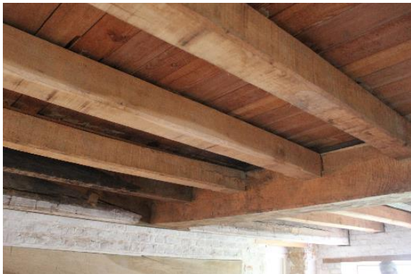
Figure 5.75, Bacon's Castle, ca. 1665 dwelling, Basement,, Room 003, view of structural members, and underside of first floor flooring.
