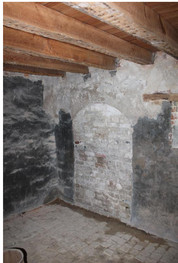
Figure 5.89, Bacon's Castle, ca. 1665 dwelling, Basement, West room, Room 005, view northwest. Note the bricked-in bulkhead door.
