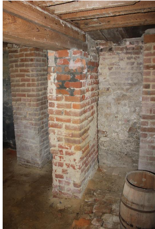
Figure 5.91, Bacon's Castle, ca. 1665 dwelling, Basement, West room, Room 005, view west. Note the modern bricks and portland cement mortar.
