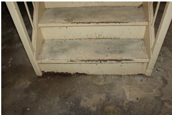
Figure 5.99, Bacon's Castle, Hyphen, Basement, Room 006, bottom treads and riser of the stair are rusty.
