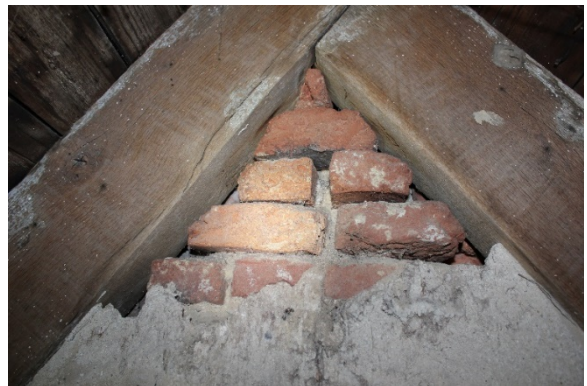
Figure 5.253, Bacon's Castle, ca. 1665 portion, Attic, Room 401, detail of the east gable peak. Note the missing mortar.
