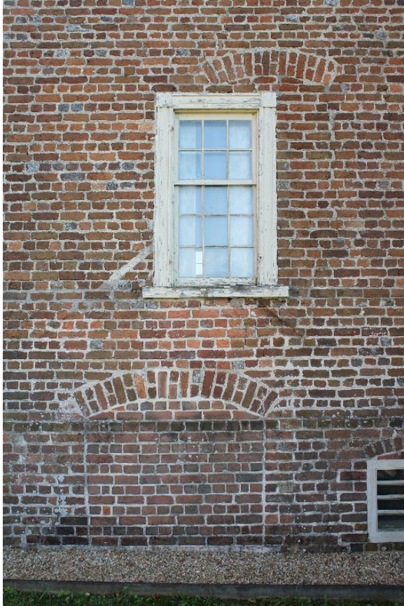
Figure 5.27, Bacon's Castle, South elevation, detail ghosting of previous porch. Note the bricked-in bulkhead door.
