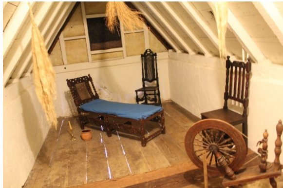
Figure 5.244, Bacon's Castle, ca. 1665 portion, Garret Floor, Room 303, detail of floor. Note the light permeating between the floorboards.
