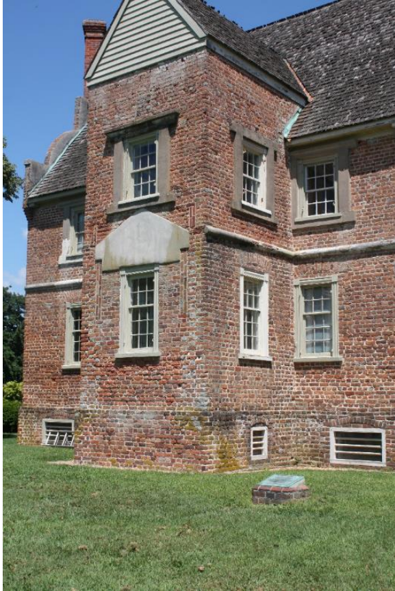
Figure 5.13, Bacon's Castle, South elevation, detail of ghosting of previous porch roof.
