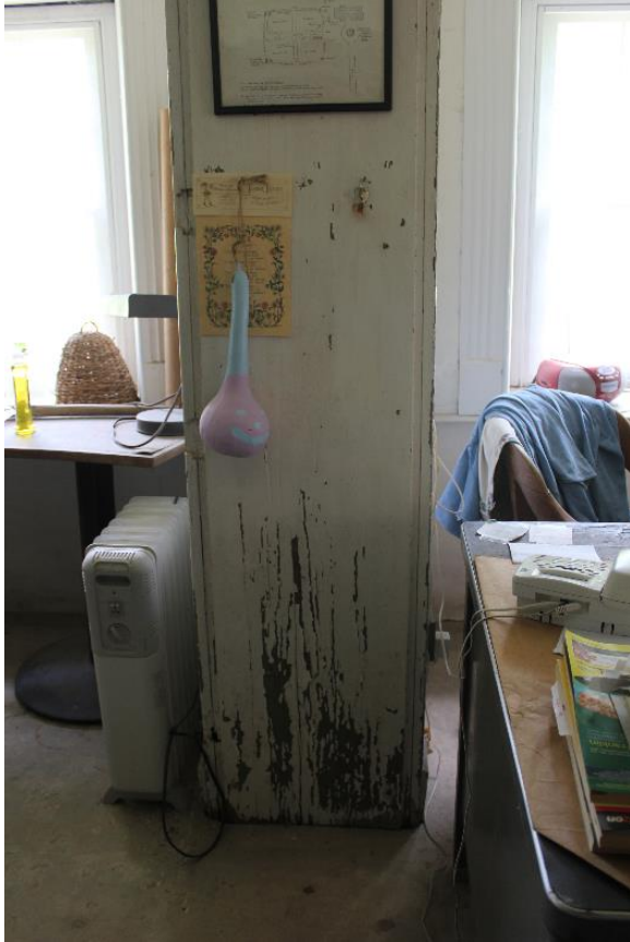
Figure 5.112, Bacon's Castle, ca. 1854 addition, Basement, Room 008,009, View east. Note the water damage at the base of the cased opening.
