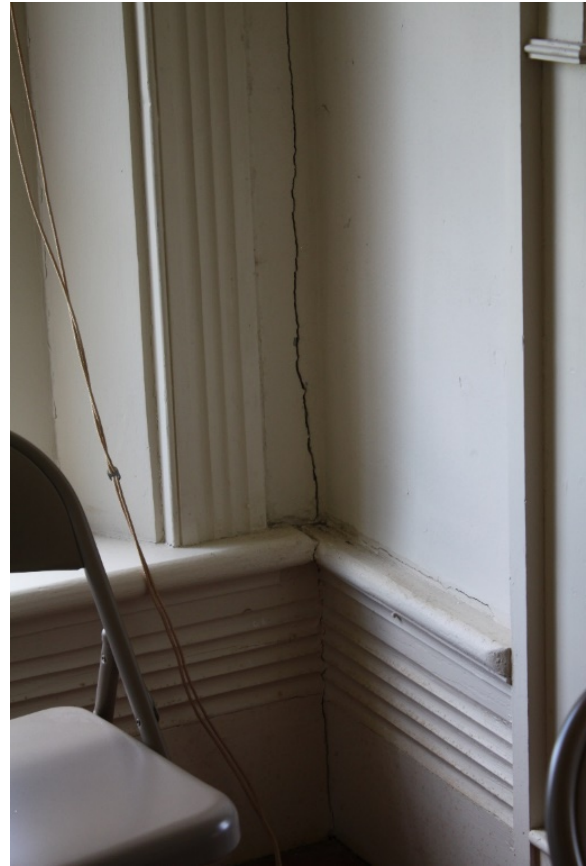
Figure 5.220, Bacon's Castle, ca. 1854 addition, Second Floor, Room 208, detail of crack in southwest corner of the room.
