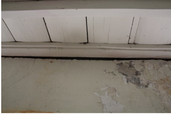
Figure 5.239, Bacon's Castle, ca. 1665 portion, Garret Floor, Room 302, detail of gap between the framing member and the chimney mass.
