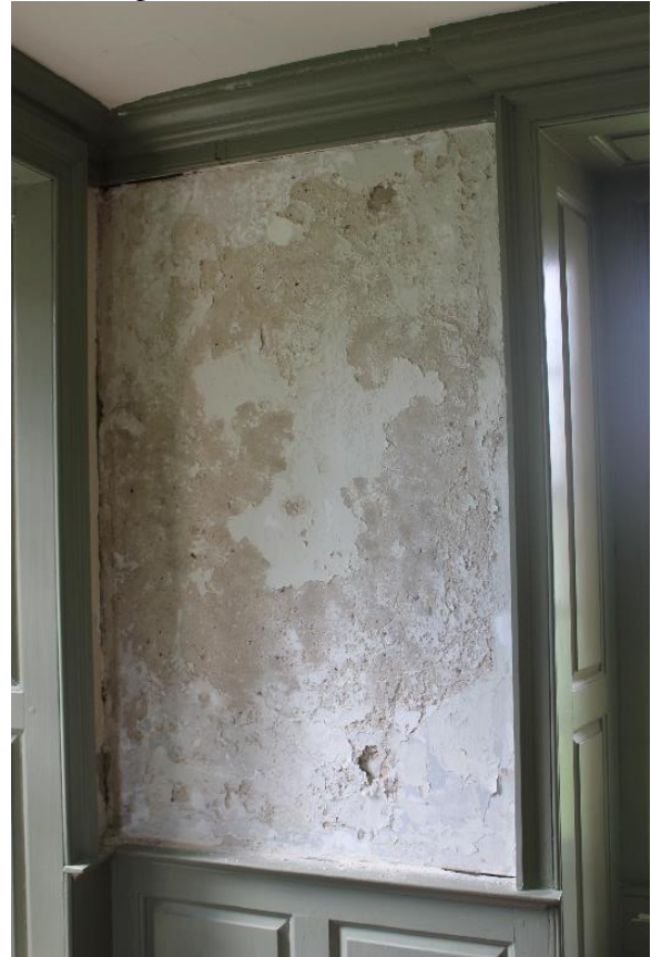
Figure 5.141, Bacon's Castle, ca. 1665 building, West Room, Room 103, detail of wall, view northwest. Note extreme efflorescence.
