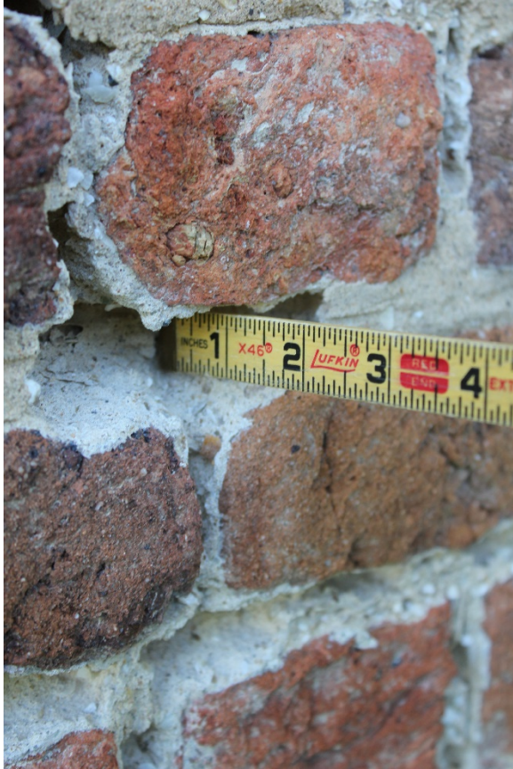
Figure 2.125: Bacon's Castle, South elevation, restoration repointing failure. Commonwealth Architects, 16 July 2016.
