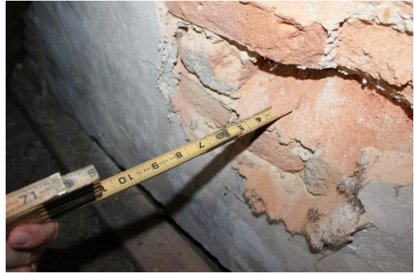
Figure 5.255, Bacon's Castle, ca. 1665 portion, Attic, Room 401, detail of the west gable wall. Note the crumbling brick. The carpenter rule was inserted four inches into the brick. This is also the location where daylight is visible through the brick wall.
