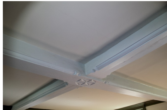
Figure 5.151b, Bacon's Castle, ca. 1665 building, East Room, Room 105, beam detail at center of room. Note steel angle reinforcement.
