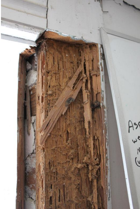
Figure 5.109, Bacon's Castle, ca. 1854 addition, Basement, Room 008,009, eastern window, south wall. Note extreme termite damage.
