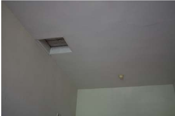
Figure 5.214, Bacon's Castle, ca. 1854 addition, Second Floor, Room 207, detail of ceiling and attic hatch.
