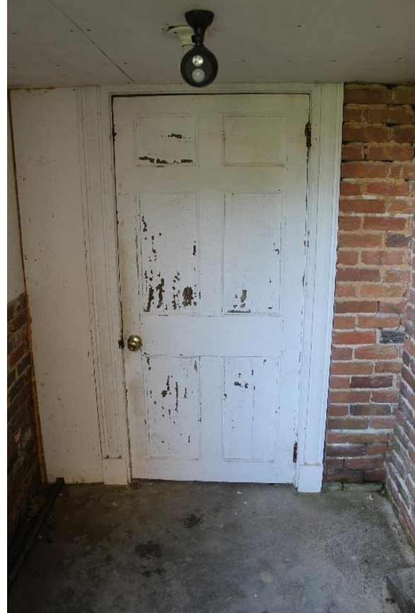
Figure 5.60, Bacon's Castle, West elevation, ca. 1950s kitchen addition, basement door. Note flaking and missing paint.
