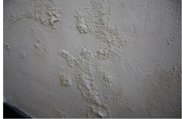
Figure 5.127, Bacon's Castle, ca. 1665 building, North Tower, Room 101, efflorescence present on the west wall.
