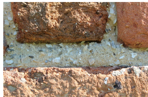
Figure 2.123: Bacon’s Castle, South elevation, restoration repointing failure; note size of aggregate. Commonwealth Architects, 16 July 2016.
