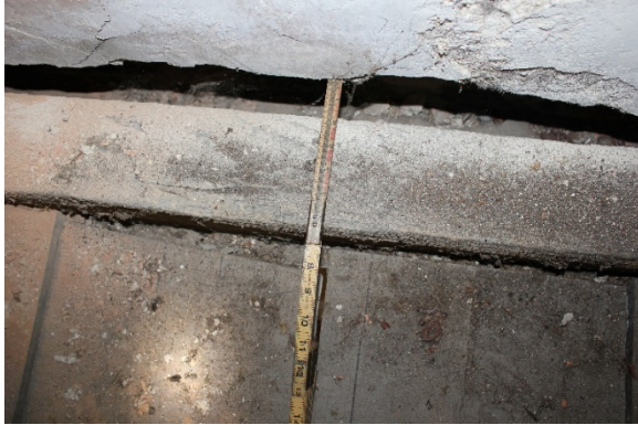
Figure 5.257, Bacon's Castle, ca. 1665 portion, Attic, Room 401, measurement of the east end wall. Note the consistent edge of the plaster at this location. Measurement taken at approximately the center of the east wall.
