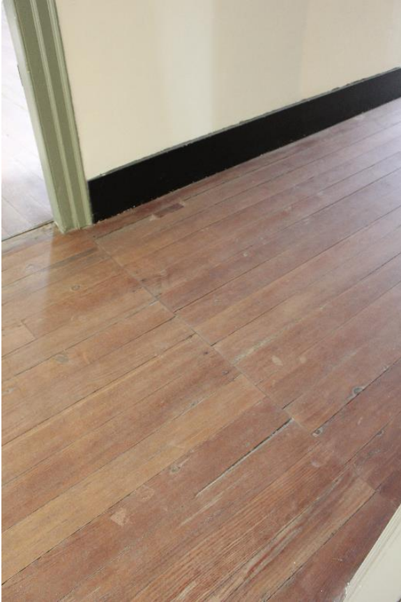
Figure 5.137, Bacon's Castle, ca. 1665 building, Corridor, Room 102 floor detail. Note the saw cut and misaligned floorboards.
