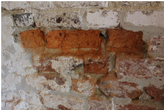
Figure 5.79, Bacon's Castle, ca. 1665 dwelling, Basement, Kitchen, Room 003, note spalled brick.
