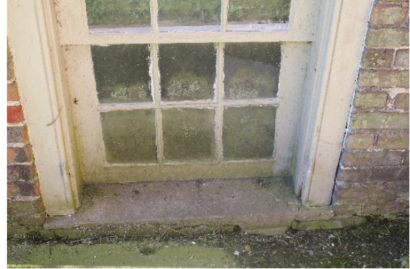
Figure 5.26, Bacon's Castle, North elevation, detail of ca. 1854 addition basement window. Note the extreme biological growth on the window frame, sash, glass, and sill.
