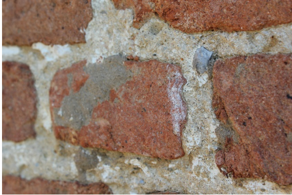
Figure 2.10: Bacon's Castle, South elevation (primary), immediately under eaves. Note irregular mortar joints, uneven brick margins, large aggregate. Photograph 26 July 2015.
