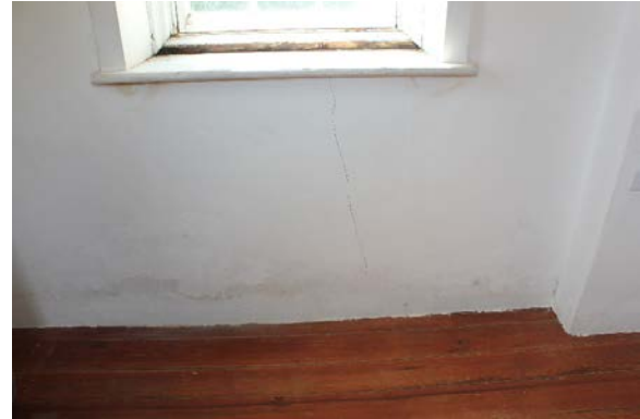
Figure 5.201, Bacon's Castle, ca. 1665 building, Second Floor, South Tower, Room 204, detail of floor and wall intersection. Note the efflorescence on the wall.
