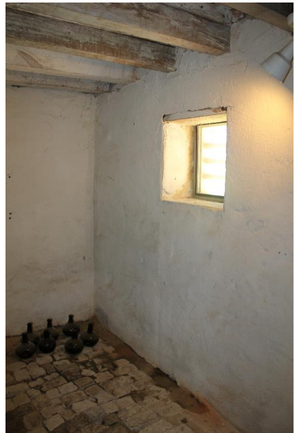
Figure 5.85, Bacon's Castle, ca. 1665 dwelling, Basement, South tower, Room 004, general view. Note the light fixture in the upper right hand corner.
