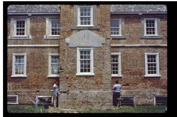
Figure 2.119: Bacon's Castle, repointing work on South elevation, 1982. Virginia Department of Historic Resources.
