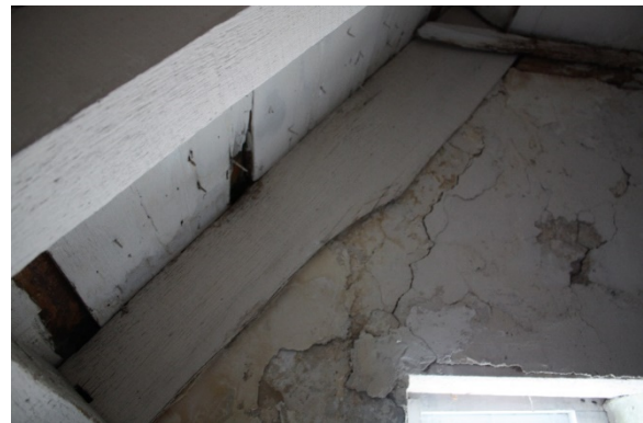
Figure 5.238 Bacon's Castle, ca. 1665 portion, Garret Floor, Room 302, detail of cracking and flaking plaster above southern window.
