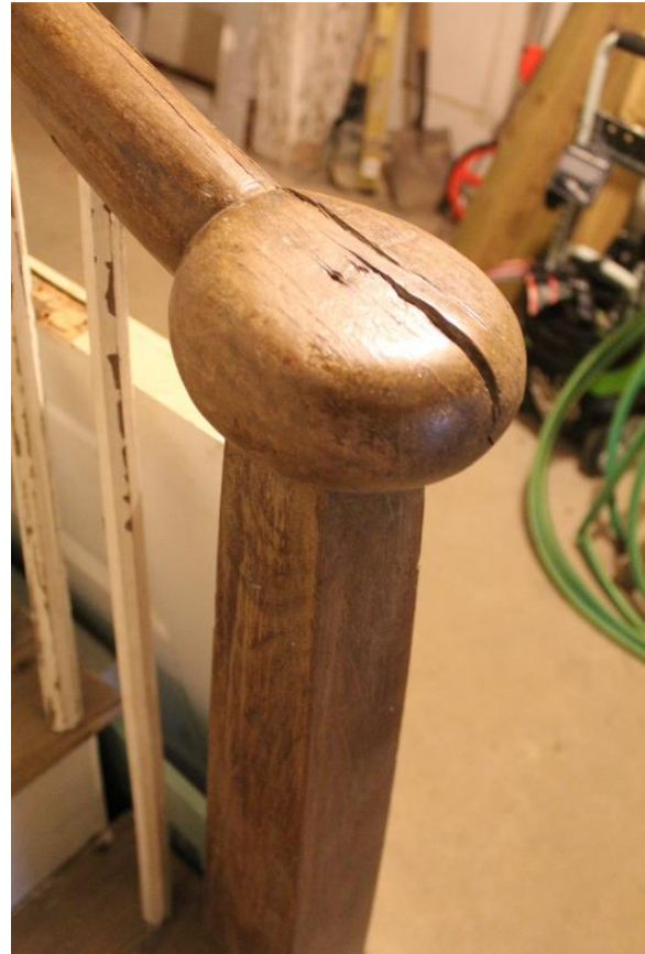
Figure 5.105, Bacon's Castle, ca. 1854 addition, Basement, Room 007, Newel post detail. Note the checking.
