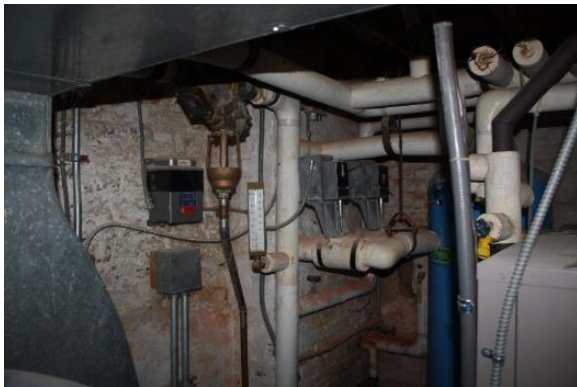
Figure 5.125, Bacon's Castle, Hyphen, Room 012, various mechanical equipment.
