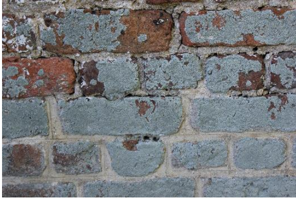
Figure 5.54, Bacon's Castle, West elevation, detail of masonry wall. Note biological growth.
