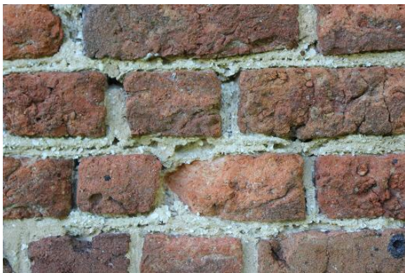
Figure 5.55, Bacon's Castle, West elevation, detail of masonry wall. Note pocked and missing mortar.
