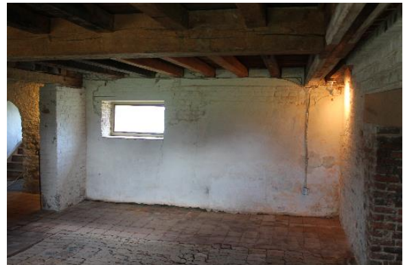
Figure 5.77, Bacon's Castle, ca. 1665 dwelling, Basement, Kitchen, Room 003, view of whitewashed brick walls and plaster. Note general mortar loss.
