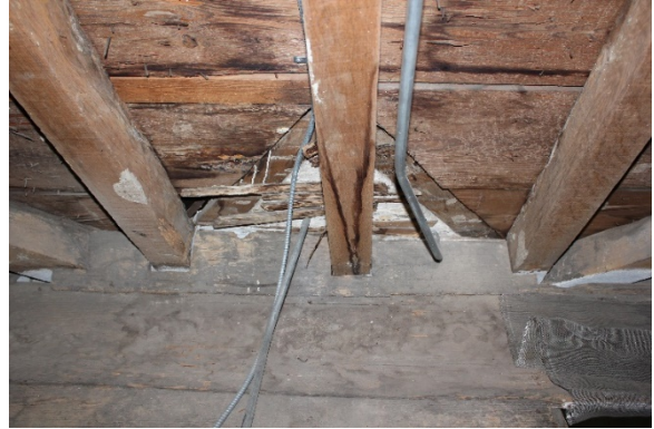
Figure 5.251, Bacon's Castle, ca. 1665 portion, Attic, Room 401, detail of the north side of the ceiling. Note the small peak of the backside of plaster on lath.
