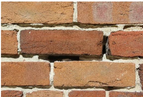
Figure 5.38, Bacon's Castle, East elevation, detail of masonry wall. Note mortar loss.
