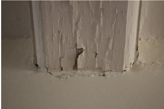
Figure 5.135, Bacon's Castle, ca. 1665 building, Corridor, Room 102, beam detail, note the cracking and flaking paint.
