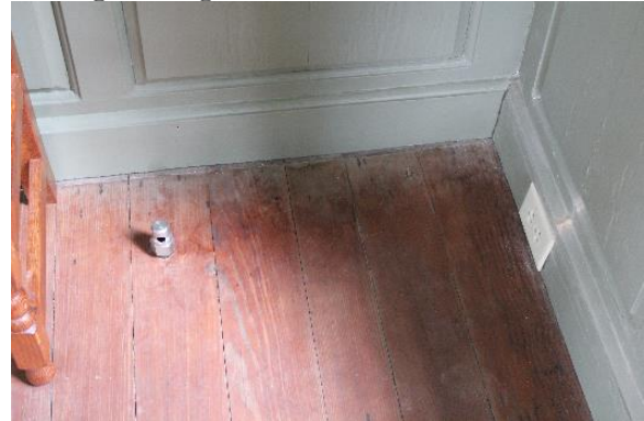
Figure 5.145, Bacon's Castle, ca. 1665 building, West Room, Room 103, detail of floorboards. Note the Halon dispenser, brick and mortar duct above the outlet, and the water damage on the floor.
