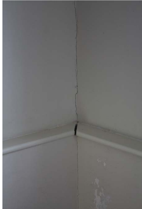
Figure 5.216, Bacon's Castle, ca. 1854 addition, Second Floor, Room 207, detail of wall and trim separation.
