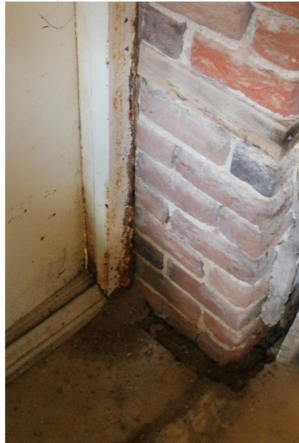
Figure 5.104, Bacon's Castle, ca. 1854 addition, Basement, Room 007, Note the rust on the door frame and door panel.
