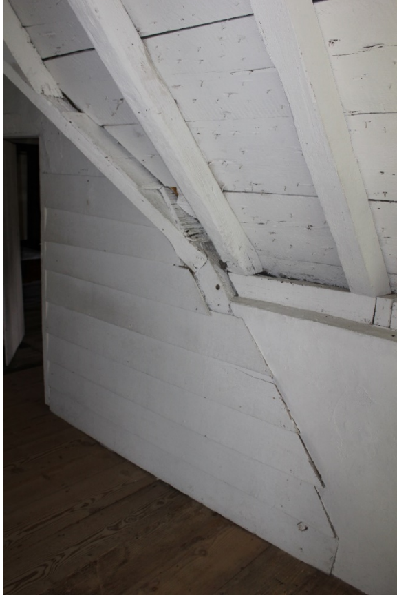
Figure 5.233, Bacon's Castle, ca. 1665 portion, Garret Floor, Room 301, detail of clapboard and plaster wall intersection.
