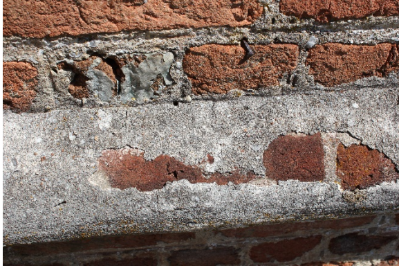
Figure 2.15: Bacon's Castle, South elevation (primary), stringcourse with some surviving oyster-shell stucco parge coat. Photograph 26 July 2015.
