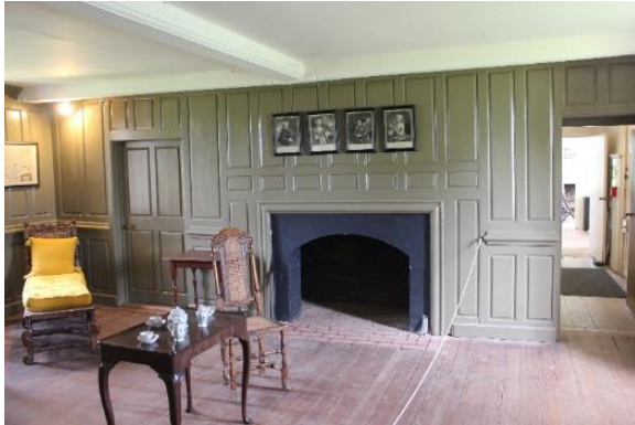
Figure 5.149, Bacon's Castle, ca. 1665 building, East Room, Room 105, general view northeast. Note the deflection of the beam above the fireplace.
