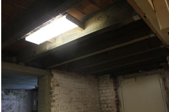
Figure 5.98, Bacon's Castle, Hyphen, Basement, Room 006, View of ceiling joists, whitewashed walls, and fluorescent light fixture.
