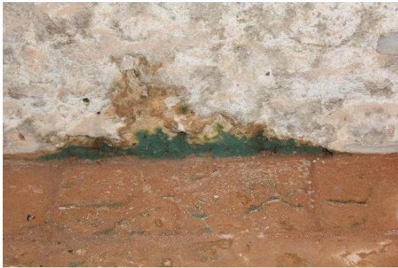
Figure 5.78, Bacon's Castle, ca. 1665 dwelling, Basement, Kitchen, Room 003, note biological growth.
