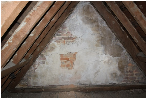
Figure 5.254, Bacon's Castle, ca. 1665 portion, Attic, Room 401, view west of west gable end wall. Note the amount of missing parge coat is greater on the west gable end wall.
