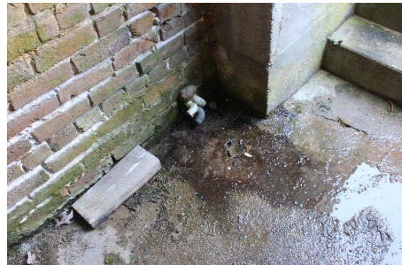
Figure 5.116, Bacon's Castle, ca. 1950s addition, Basement, Room 010, note condensate drainage and biological growth.
