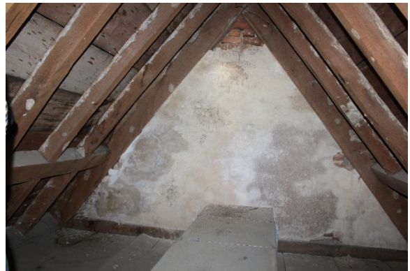
Figure 5.252, Bacon's Castle, ca. 1665 portion, Attic, Room 401, view east of east gable end wall. Note the missing coat and the large duct.
