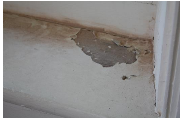
Figure 5.148, Bacon's Castle, ca. 1665 building, South Tower, Room 104, window sill detail. Note the flaking paint and brick and mortar dust.
