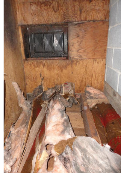
Figure A68: Deteriorated west wall and coal chute.
