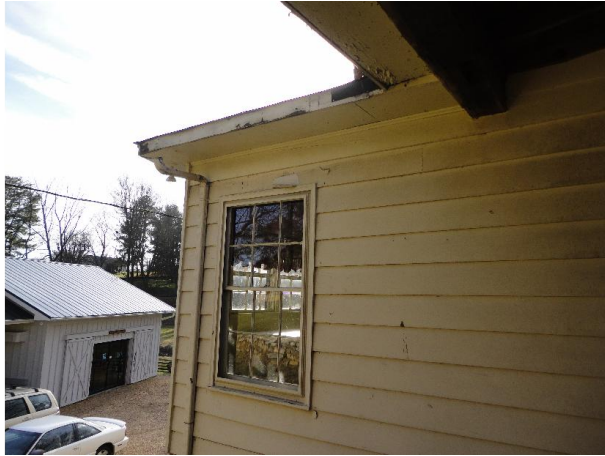
Figure A42: Typical pressed wood siding rot and paint failure.
