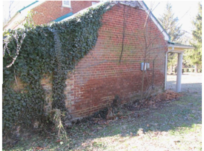
Figure S16: Rising damp at east wall of Judge's Chambers
