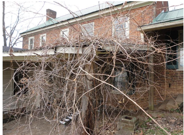
Figure A41: Rot at patio supports.
