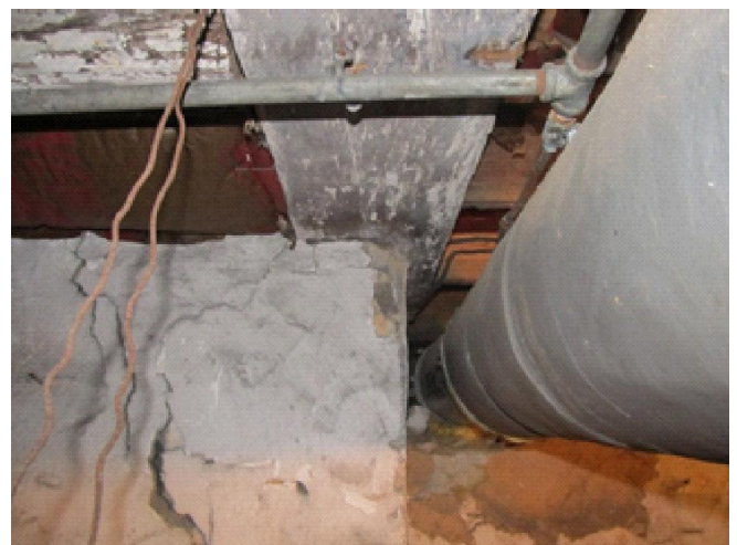
Figure S9: Floor Separation
