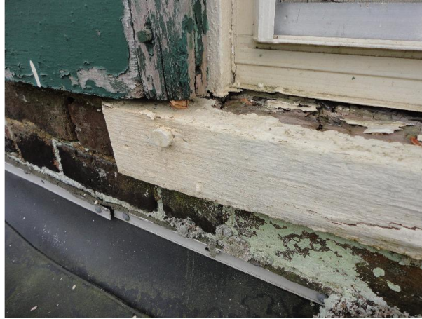
Figure A58: Sill Rot at W201.
