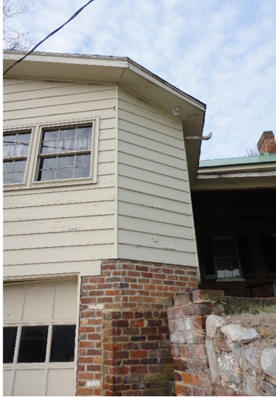
Figure A66: Missing rainwater leader at south façade.
