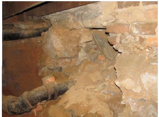
Figure S5: Pipes at access door at northwest corner of Retirement I.
