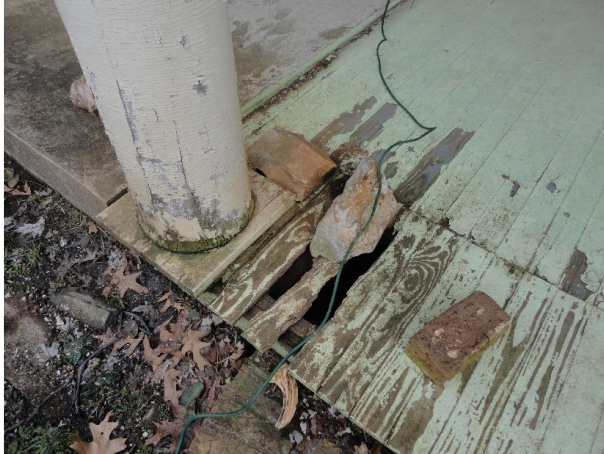
Figure A64: Rotted porch columns and flooring:
