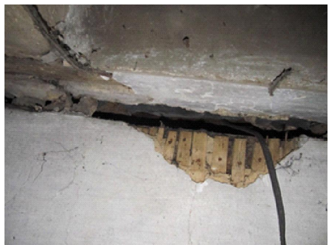
Figure S6: Bearing post condition.
