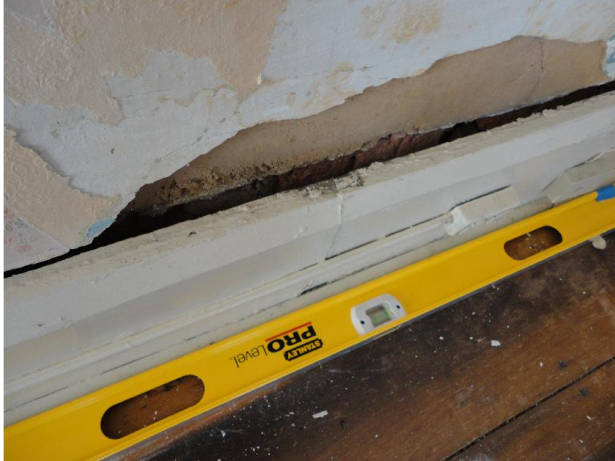
Figure A75: Separation at south wall of Bedroom 202.
