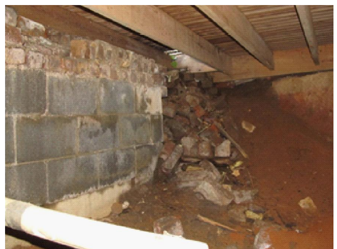
Figure S3: Foundation wall at front porch
