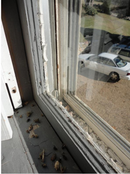
Figure A57: Putty Failure at W114.
