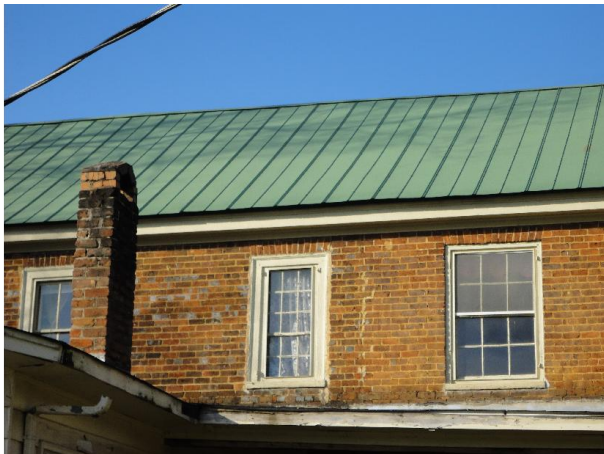
Figure A40: Visible joint between Retirement I and II.
