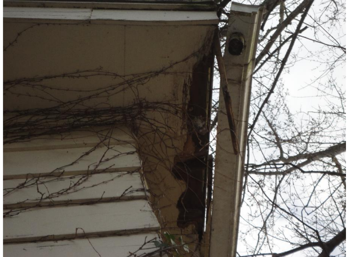
Figure A45: Rot at rear addition soffit and fascia.
