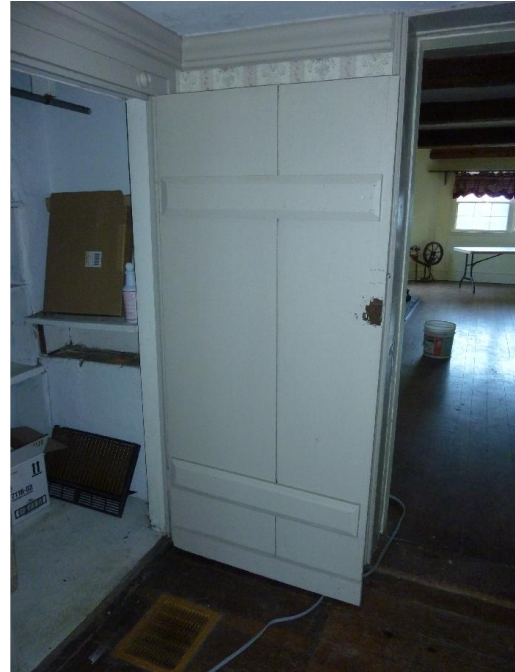
Figure A20: Sill of Retirement I window visible in closet below stairs.
