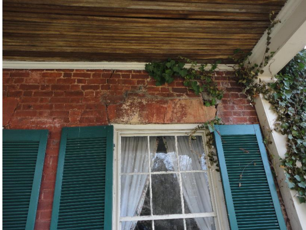
Figure A36: Lintel cracking at Northwest corner.
