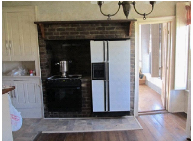
Figure S17: Unsupported brick fireplace, removed February 2014
