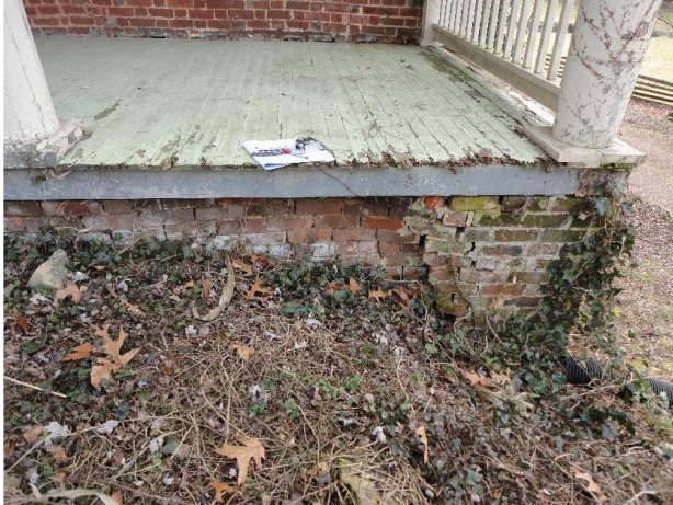
Figure A69: Brick foundation failure at northwest corner of front porch.
