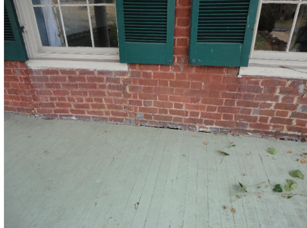
Figure A37: Sill cracking at Northwest corner.
