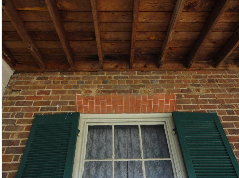
Figure A28: Brick tinting and mortar joint chalking at the south facade.
