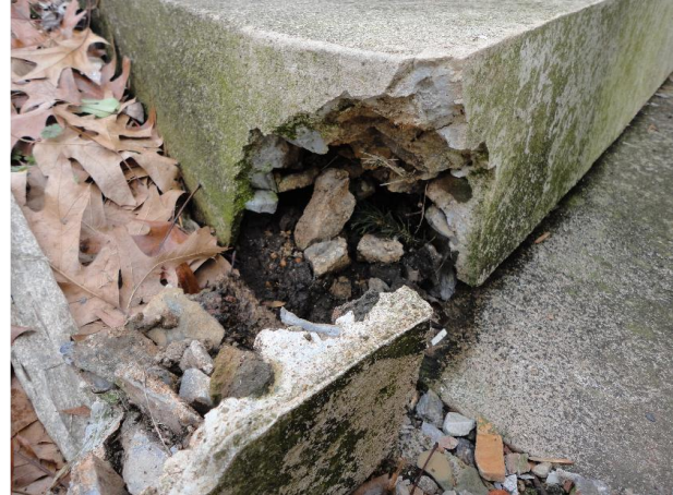
Figure A65: Failing concrete step at curving concrete stair from Main Porch to Judge's Chambers Porch.
