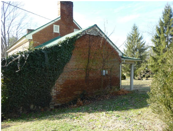
Figure A38: Rising damp at east facade.
