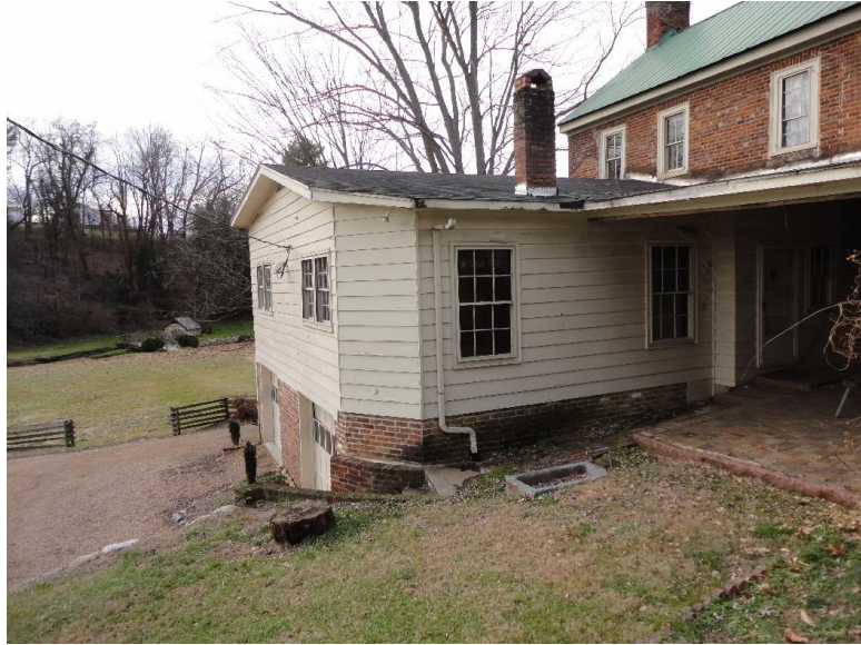
Figure A26: Evidence of the former peak of the rear addition roof visible in the masonry wall at the western window.
