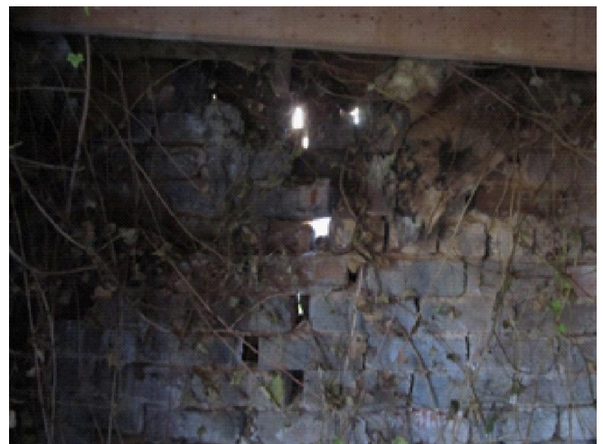
Figure S2: Foundation wall at front porch
