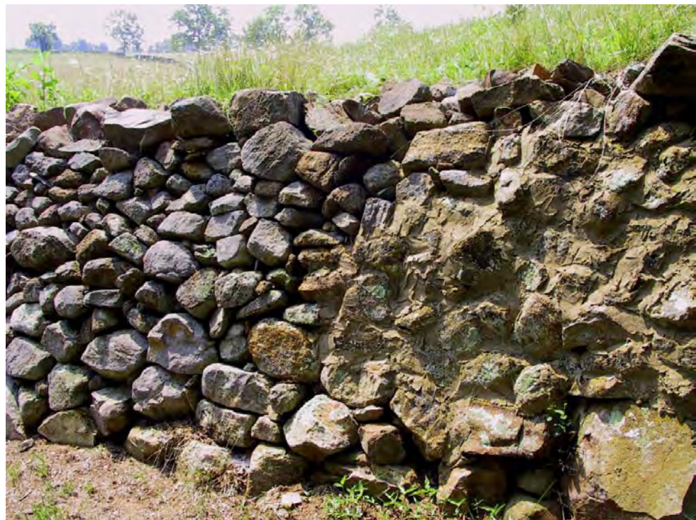
Figure 66. Retaining wall just south of Running Brook farmhouse. Originally drylaid, a portion (right) has been reinforced with mortar.
