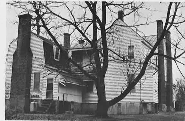
BOYKIN'S TAVERN, ISLE OF WIGHT COUNTY: The only surviving structure associated with the Isle of Wight County courthouse of 1800, the tavern was built for Colonel Francis Boykin who was instrumental in arranging for the removal of the court from Smithfield.
