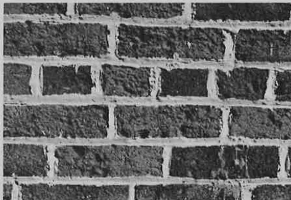
Early-nineteenth-century brickwork that has been sandblasted and repointed with no care taken to match the original joints.
