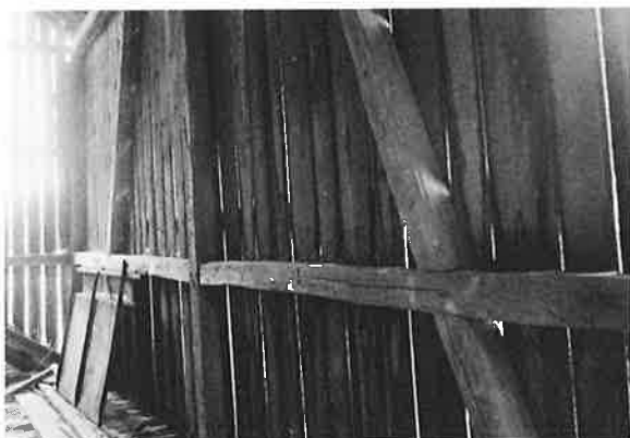
Interior detail of Christian-Brown Barn showing plate to sill bracing and horizontal rail.
