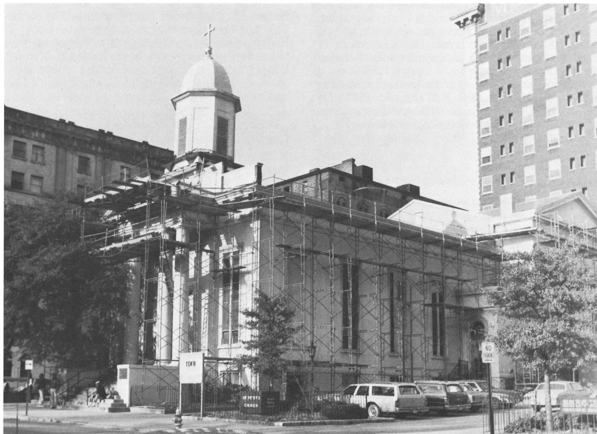
Work is proceeding on Jobs Act project at Saint Peter's Church, Richmond.
