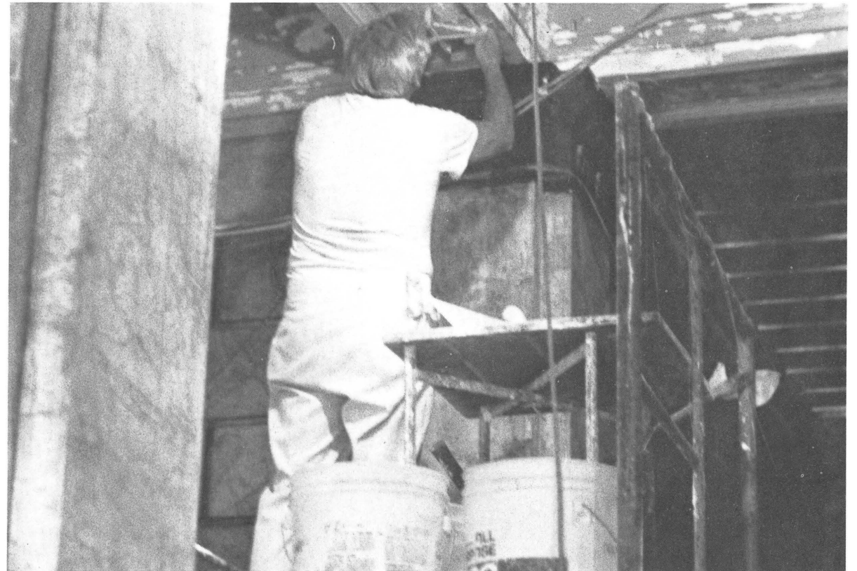
Plasterer working on ceiling in the Jefferson Hotel, Richmond. This project is slated for completion this winter.
