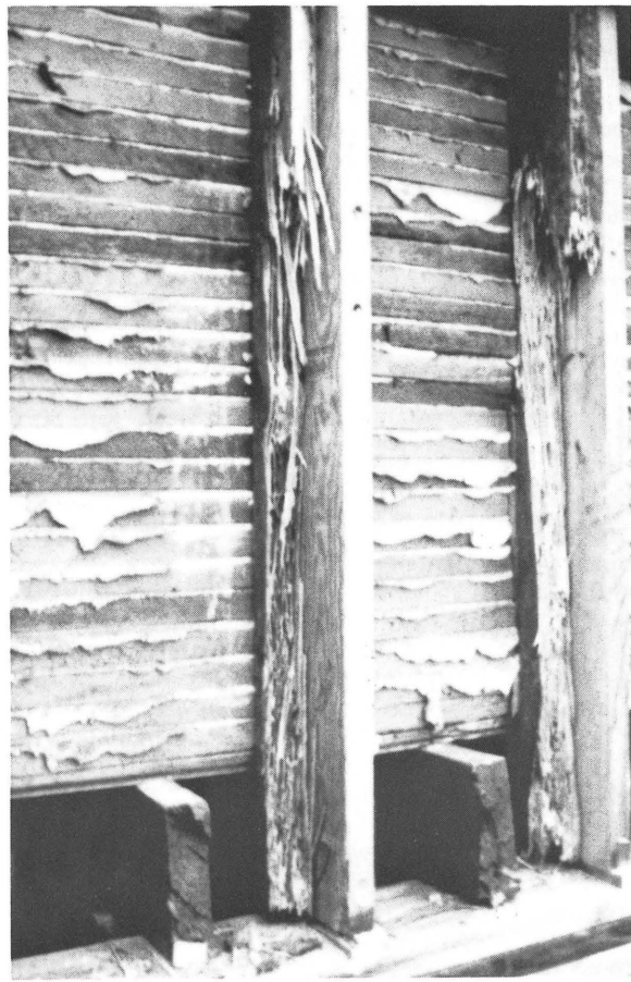
Plate Number Five: Structural deterioration uncovered during restoration, showing rotted studs scabbed with replacement studs.
