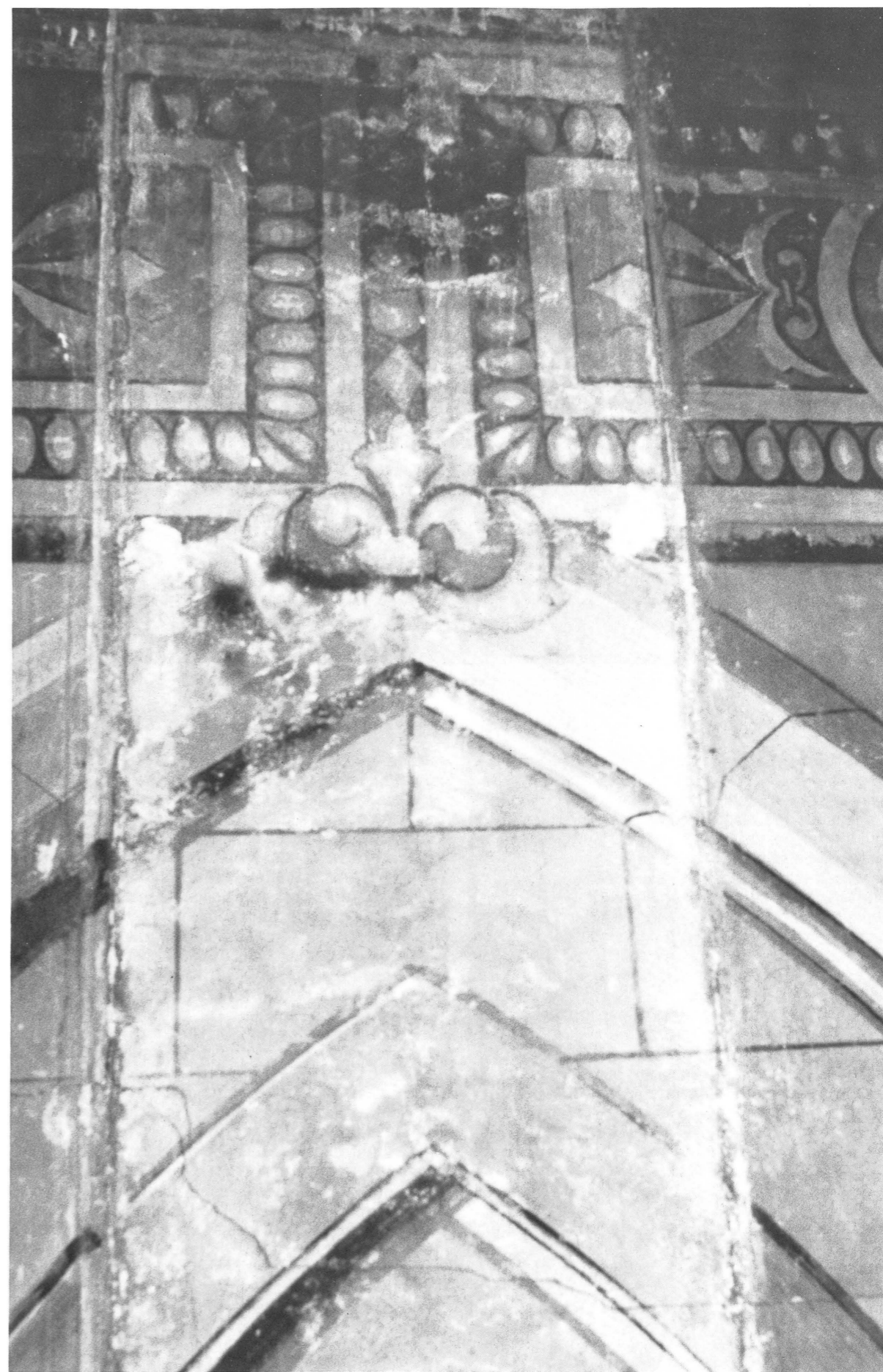
Plate Number Nine: Ghosting of original murals after removal of concrete block chimneys in sanctuary.
