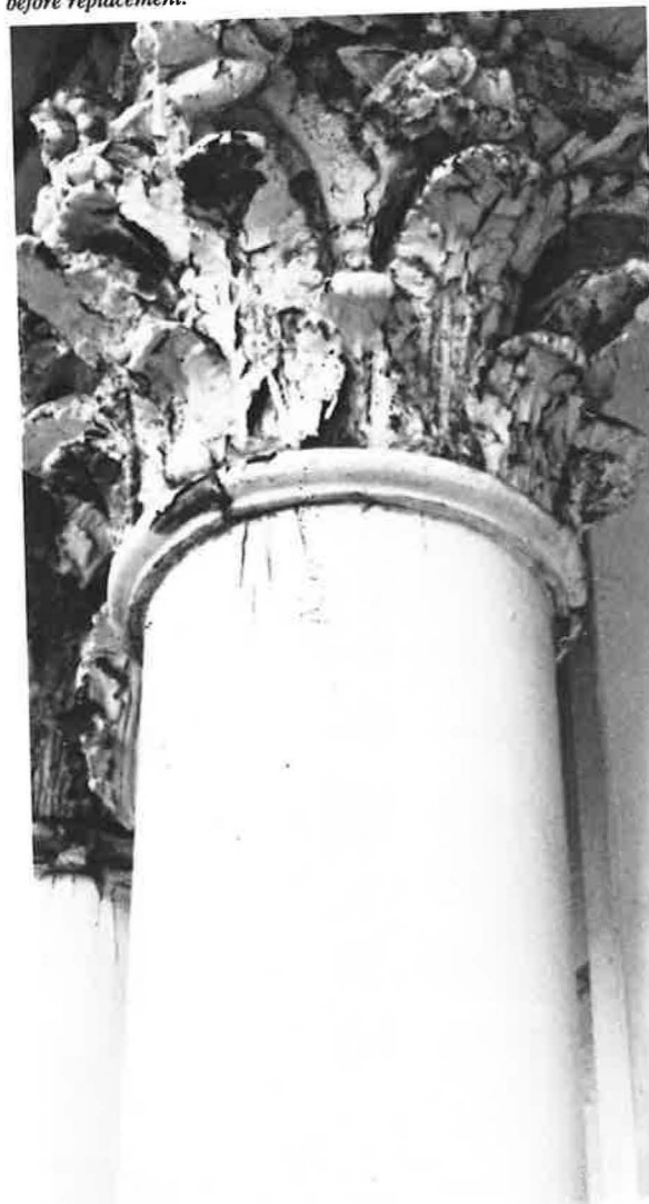
The capitals on the front elevation of the Alexander Baker House before replacement.
