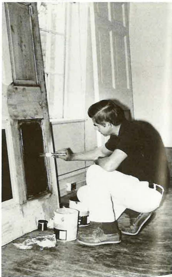
Andy Johnson, restoration expert for Monticello, instructed two University painters in the techniques of graining required for doors in each of the ten Pavilions.
