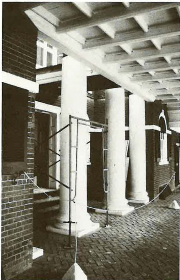
As had been the case in the early 19th century, light once again spills over the edge of the colonnade deck, following removal of closures made during the 1850s.
