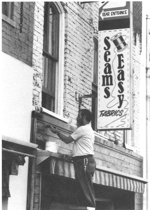
This store has been in continuous use as a commercial structure since it was constructed in 1920. The exterior renovation was completed in November 1986 following the design work and specifications prepared by Kathy Frazier. City of Bedford.
