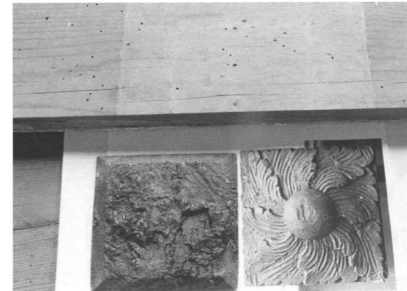
Plank from original Doric frieze showing spacing of triglyphs and metopes. Plank was discovered when researchers dismantled the wall beside the entrance doorway.
