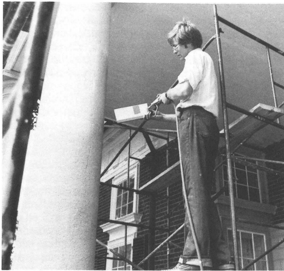
To create a replication of the original sandstone finish on the East Portico columns, sand was sprayed on to wet paint with a trough and air compressor nozzle. Credit: Frank S. Welsh
