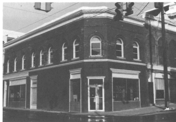
102-106 N. Bridge Street. The brickwork has been chemically cleaned, the masonry has been repaired and the wood trim has been repaired.
