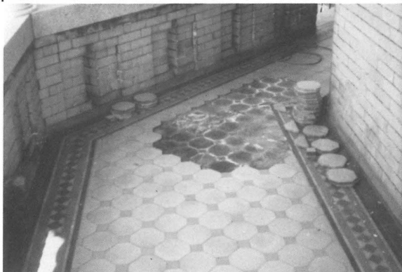
Rehabilitation of the front porch of the High Street Inn in progress; regrouting and repair of polychromatic tile. Petersburg.
