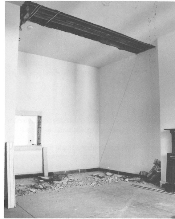
Katherine Wetzel, photograph, Jefferson Davis's Office, 1987. The removal of ceiling plaster in Davis's second floor office revealed double joists indicating the location of a partition wall in place during the Davis occupation. The small room created by the partition wall served as the office of Davis's secretary, Burton Harrison.
