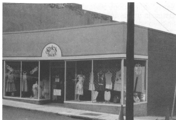
202 East Washington Street showing new stucco over concrete block, new paint, signs, and graphics.
