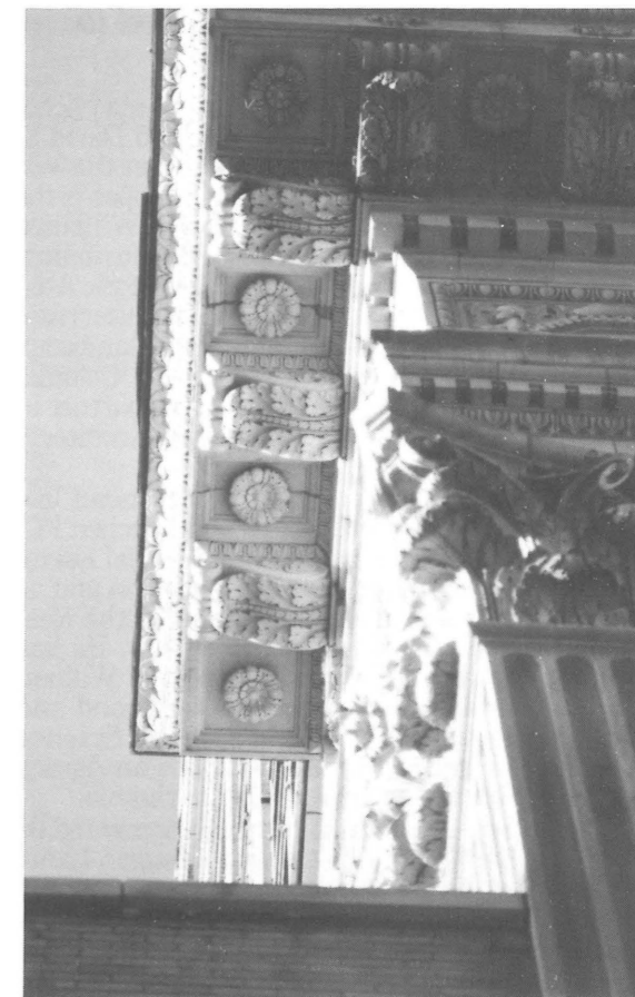
First National Bank Building, 823 East Main Street, Richmond. Close-up, terra cotta ornament on south elevation. Credit: DKM Richmond Associates.
