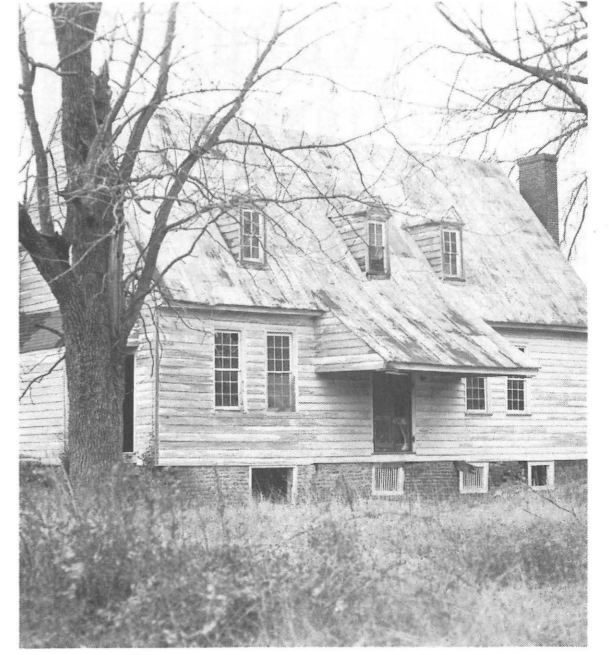
Doswell, an abandoned farmhouse in rural Hanover County that will be surveyed with help from the grant from the Division of Historic Landmarks.
