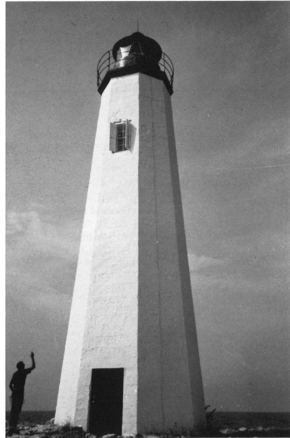
The New Point Comfort Lighthouse in Mathews County after the exterior stone masonry was hand scraped and repainted white.
