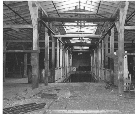
15-23 N. Nineteenth Street, Superior Industrial Machine Complex, Shockoe Valley and Tobacco Row Historic District, Richmond, before rehabilitation.
