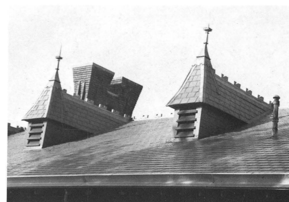
Reconstructed dormers and chimneys have returned the roof of the Pulaski Passenger Depot to its original appearance.
