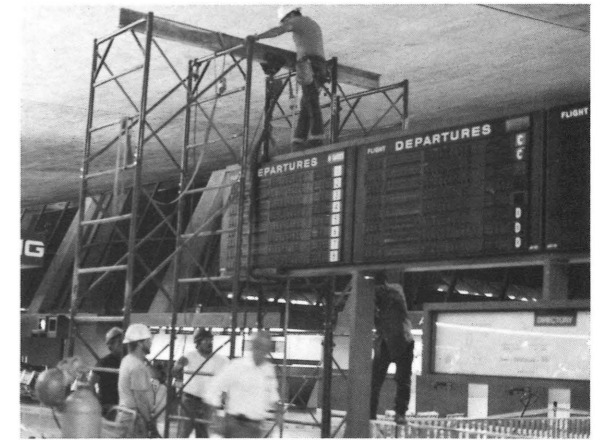
The Solari boards are taken down from their strategic place in the main terminal at Dulles International Airport.
