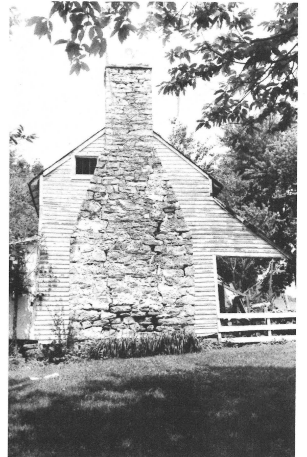
Stone chimney on detached kitchen of the Anderson House, Catawba Valley, Roanoke County.
