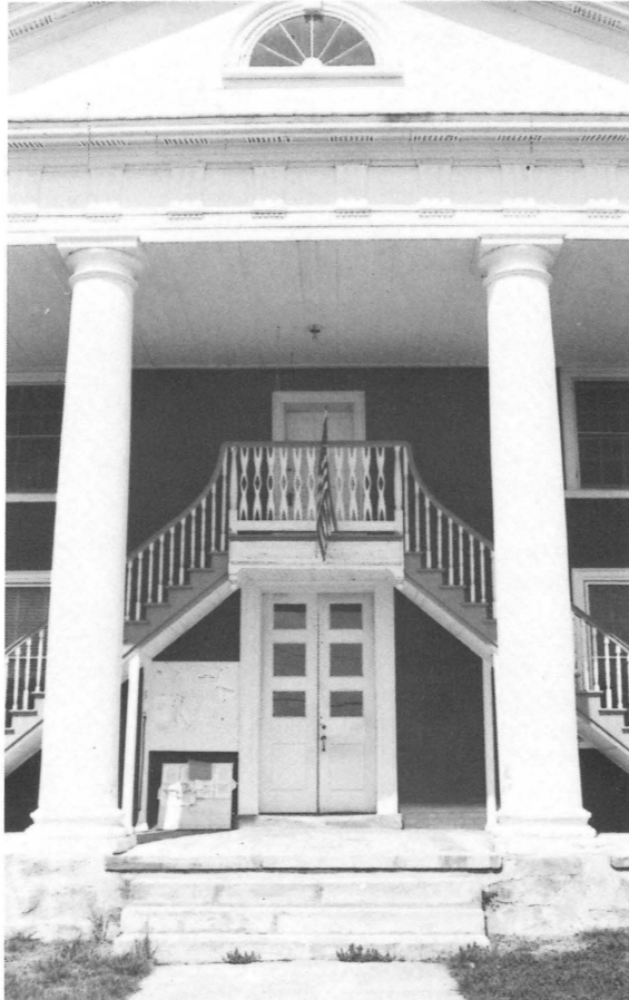
The character-defining features of the Lunenburg County Courthouse will be preserved during its renovation.
