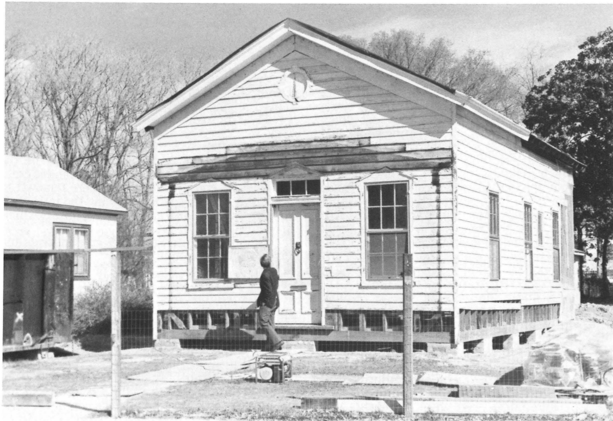
The distinctive features of St. Dennis' Chapel in Hopewell's City Point Historic District were revealed when an early porch and siding were removed.
