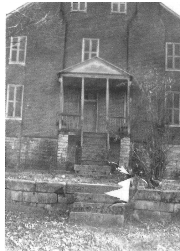
Brook Hall, Washington County, needing extensive rehabilitation.
