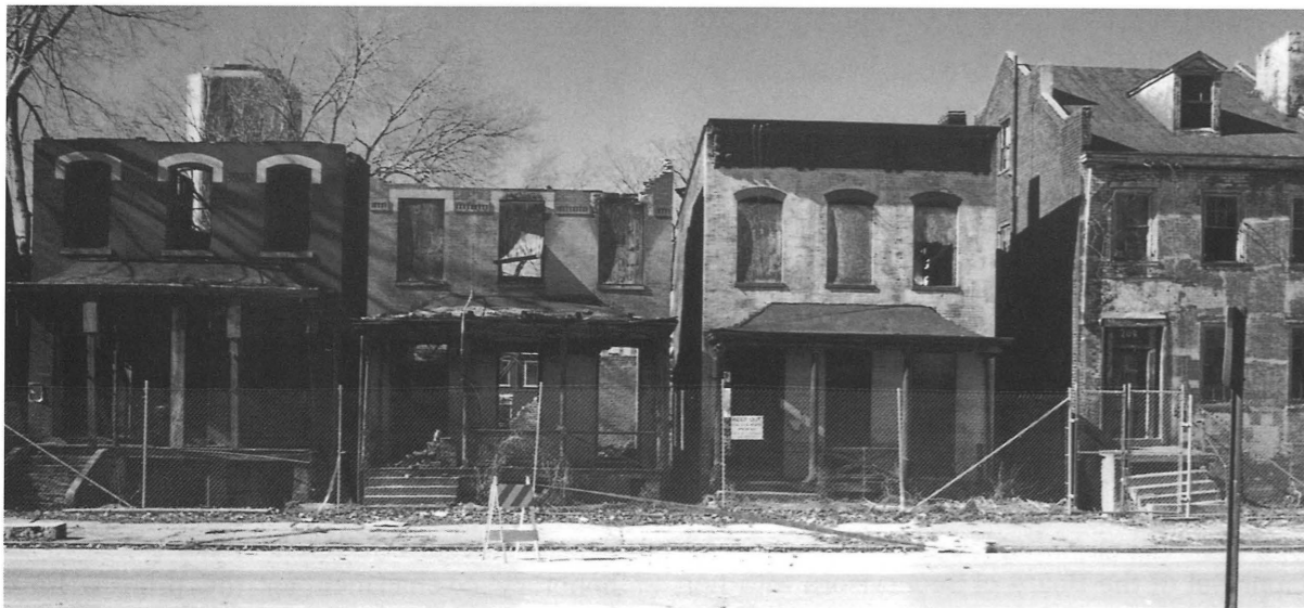
In Your Ear rehabilitated these dilapidated row houses in Richmond (above) into a cutting-edge recording studio (next page). Behind the seemingly separated facade now lies the 18,000-square-foot studio.
