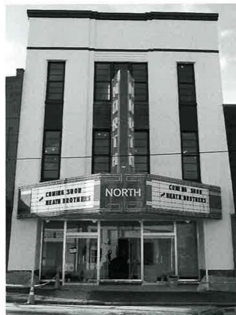
The North Theater after restoration of its marquee, windows, and façade to their 1947 configuration. The theater's historic interior features include decorative trim and light fixtures, terrazzo flooring, and lobby and balcony stairways with metal balustrade.
