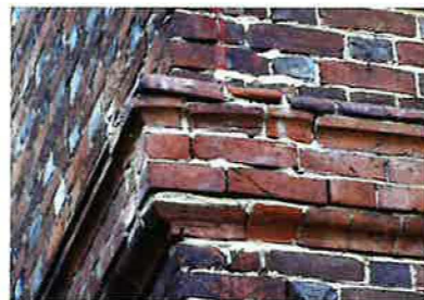
The stringcourse that encircles the mansion between the first and second stories is formed using three types of uniquely shaped, cut-and-rubbed bricks. The section of the stringcourse shown here was severely damaged when a downspout was installed decades ago. It was repaired improperly when the downspouts were removed but is now being properly restored by Bill Payne, using bricks made with clay from the plantation. (Photo: Author)
