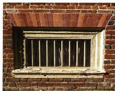
This basement window header, called a jack arch or flat arch, clearly shown in the diagonal row of bricks above the window, was recently reconstructed by mason Bill Payne with bricks he made on the premises of Shirley. The extremely thin joints between the bricks have no mortar; instead, the sides of the bricks are buttered with a thin coat of lime putty. After the bricks were set in place, their surfaces were gently sanded to give them the same smooth appearance as the original 18th-century rubbed bricks. (Photo: Author)
