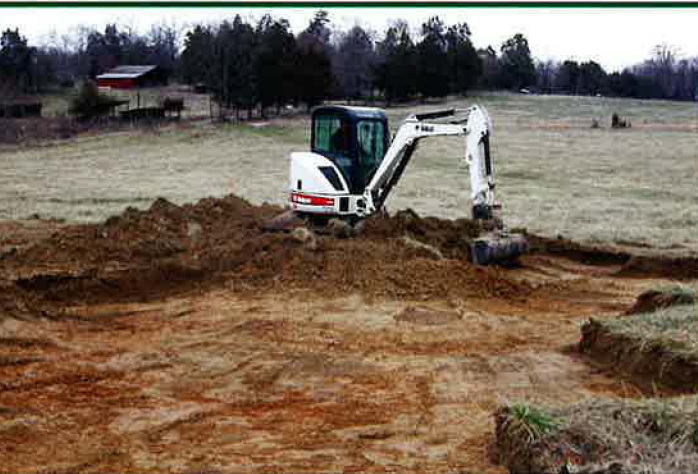
After the soldiers marched away, farmers worked the land for most of the last 145 years, and their plows created a scrambled surface layer. Operator Jeff Blankenship spent three weeks stripping that topsoil stratum from an area larger than a football field, and exposed over 500 pits from the winter of 1862-1863. (Author photo)
