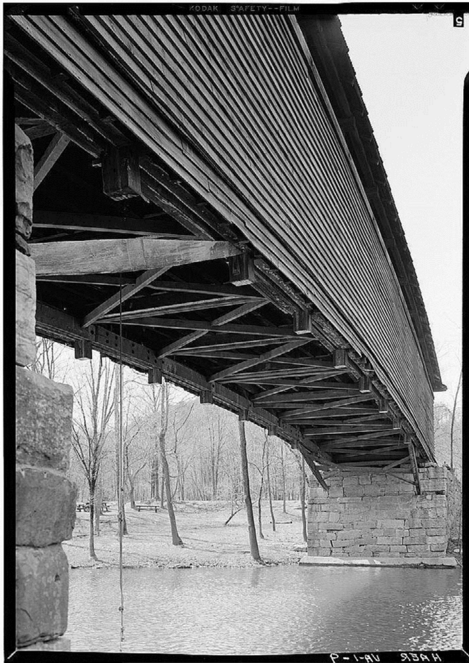
HUMPBAC BRIDGE. Abutments and floor system from southwest. Photograph by Jack Boucher, 1971
