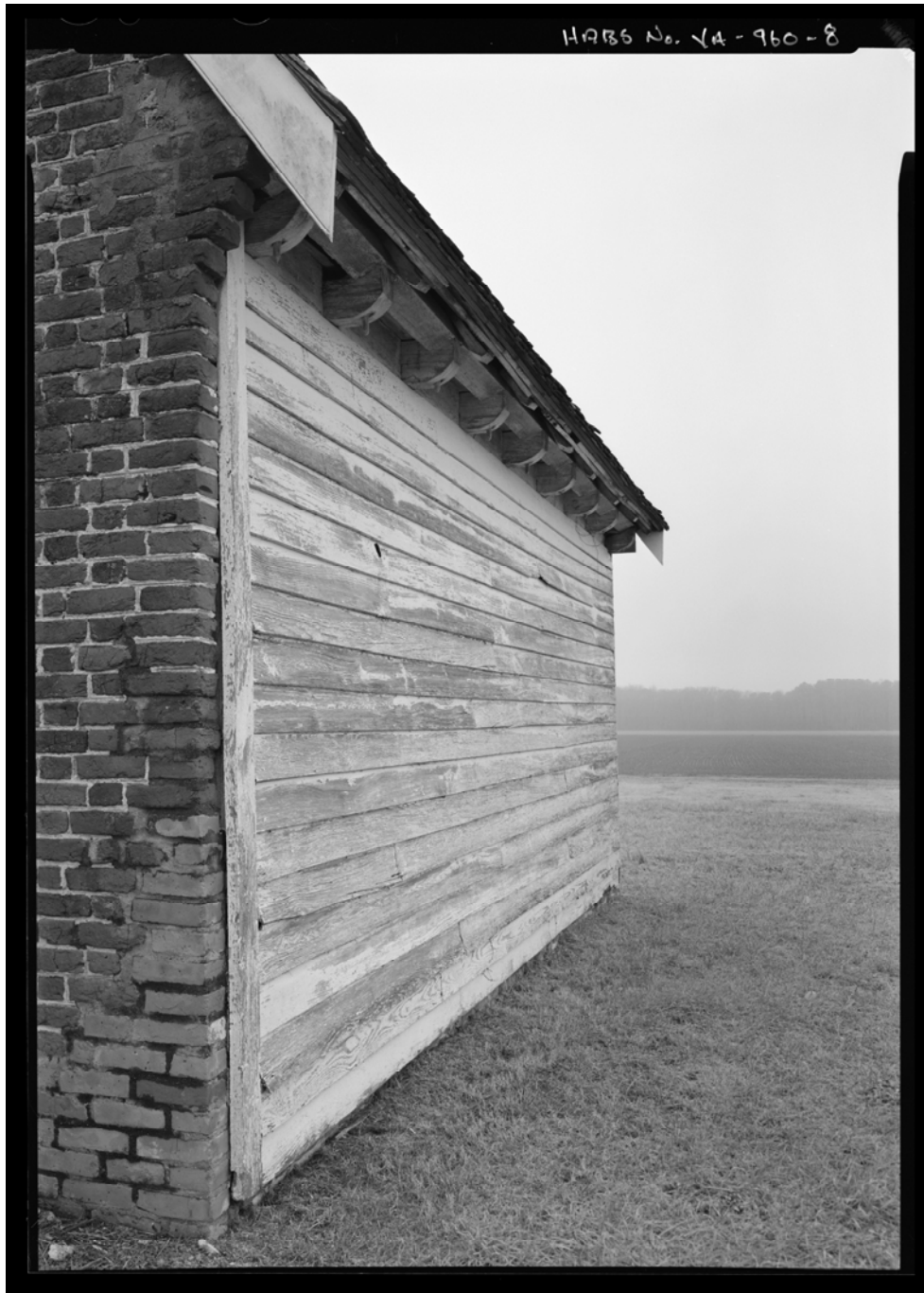
Detail view of the west elevation, showing false plate and rafter ends Photograph from HABS, James W. Rosenthal, photographer, 2011
