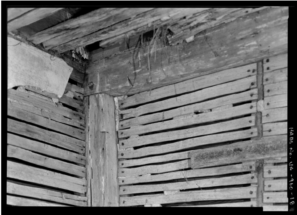
Interior view, detail view in the southwest corner to show framing; note the chamfer detail on the corner post and end girt Photograph from HABS, James W. Rosenthal, photographer, 2011
