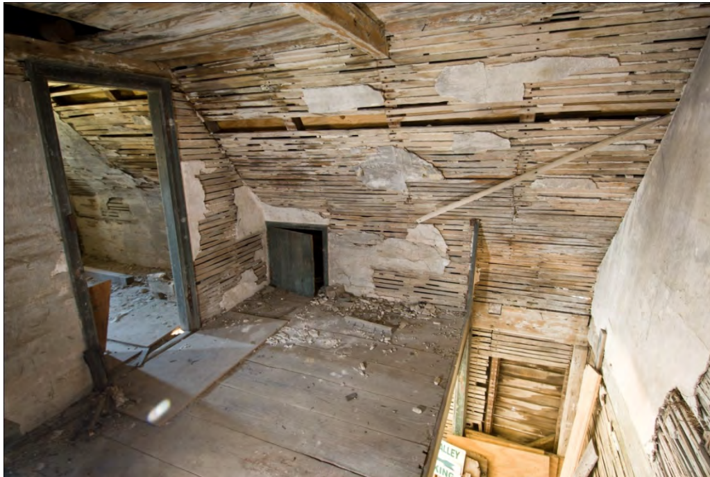
Interior view, south room of loft, looking northeast; note the knee wall door at center left Jeff Klee, Colonial Williamsburg Foundation, 2010
