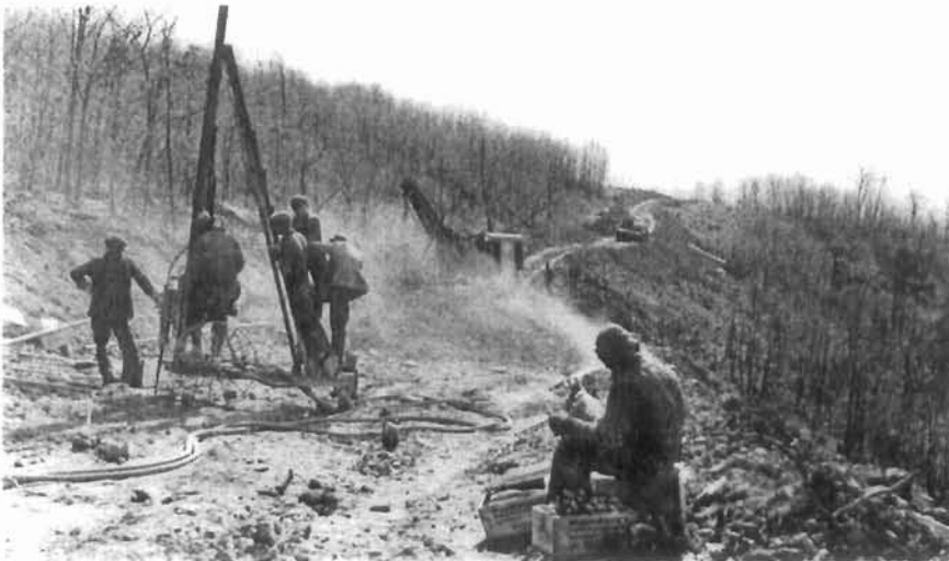
Clearing and grubbing the right-of-way for Skyline Drive, October 1934. Photograph by Lynn M. Harris. Shenandoah National Park Archives
