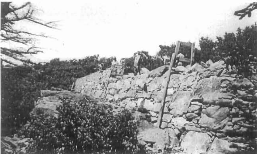
Parapet and retaining wall under construction at Crescent Rock Overlook, Shenandoah National Park Archives (no. P138b).
