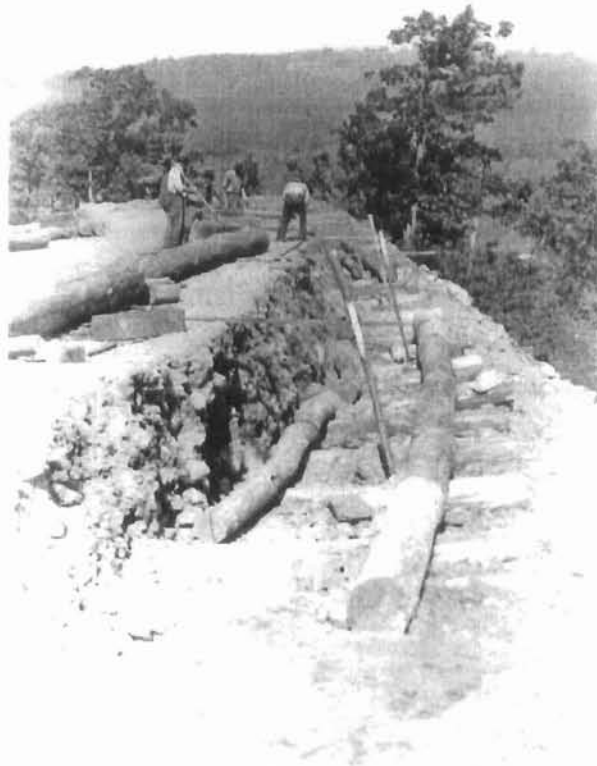
Laying cribbing on Skyline Drive near Thornton Gap, October 1933, Project 1-A. Photograph by Lynn M. Harris, Shenandoah National Park Archives (no. P198b).
