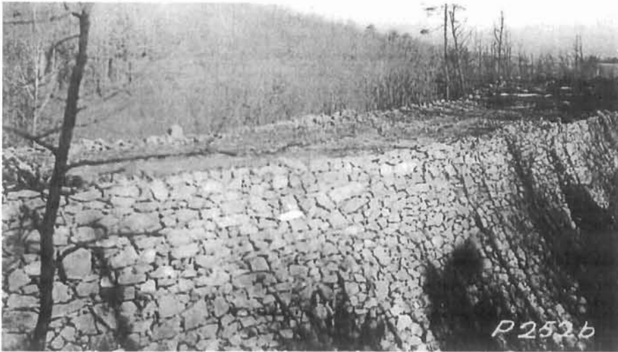
Hand-laid rock embankment at mile 1.5, Project 2-A, March 1935. Photograph By Scudder Griffing, courtesy Shenandoah National Park Archives (no. P252b).
