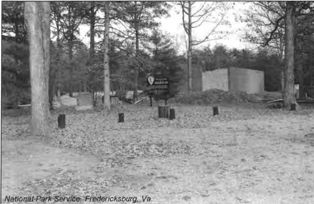
Figure 38. Chancellorsville Visitor Center, 1961 (source: Fredericksburg and Spotsylvania NMP). Photo shows Chancellorsville Visitor Center under construction; sign in the center of the image states that the project is part of Mission 66 improvements.
