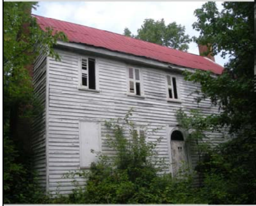
Thornton House, Halifax County, ca. 1833, deteriorating condition but retains integrity. Listed under Criteria A and C
