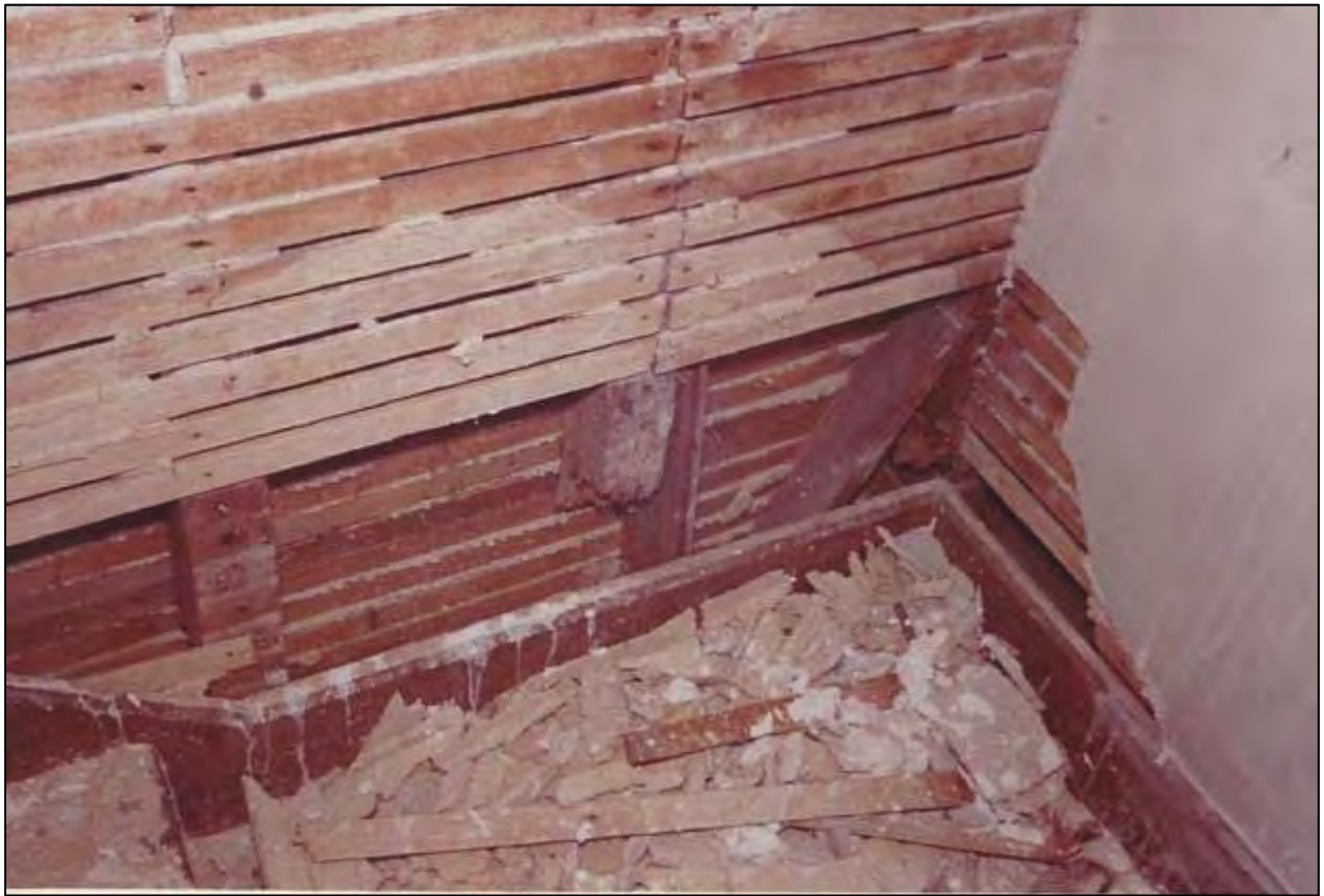
Historic Photo 4 of 5 Detail of stair landing between first and second stories: stud splintered in 1865 shelling
