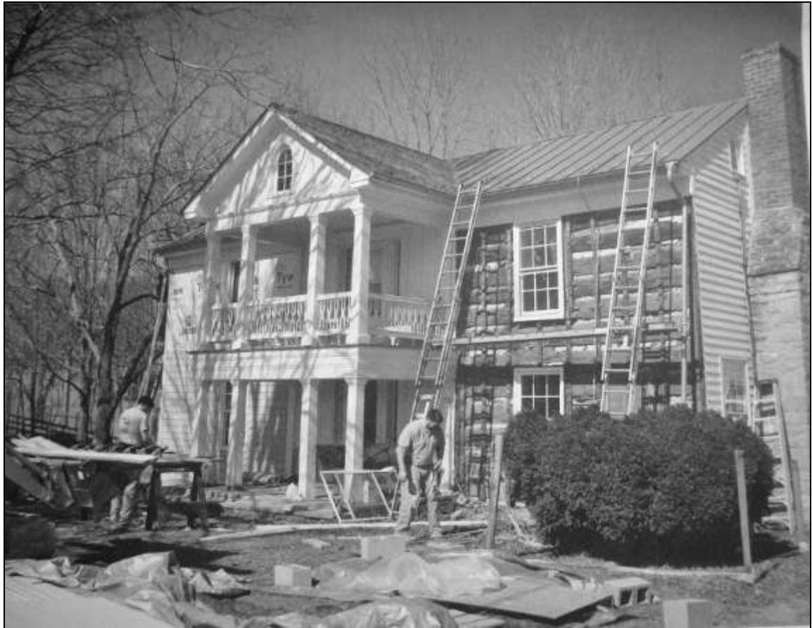
11. Slusser-Ryan House during Renovation Showing Log Construction of East Wing, Prior to 2011. Source: Susan Bull Ryan.
