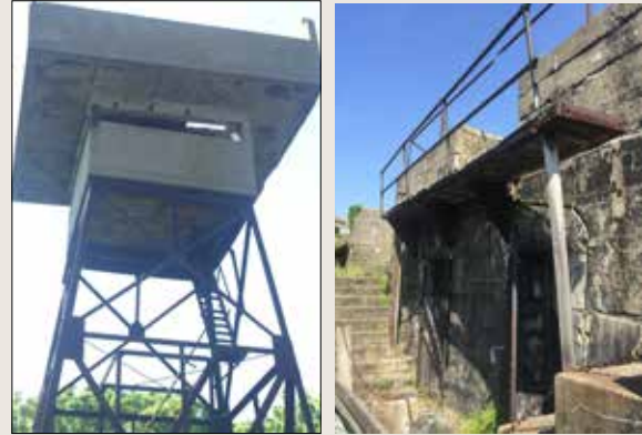
A collapsing World War II tower and a buckling wall.
