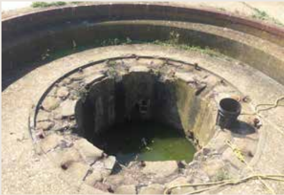
A plugged drain needing cleaning out.
