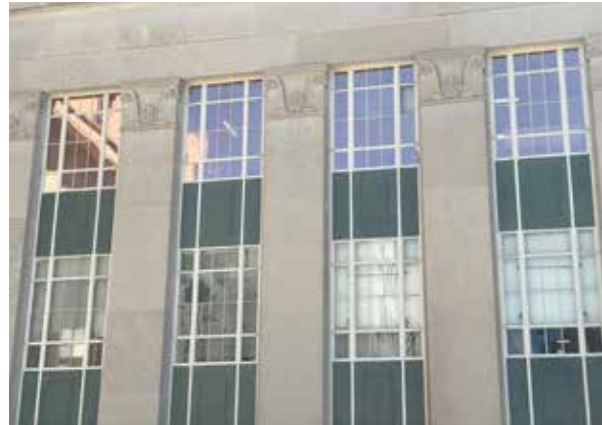
Top: VDOT's Central Highway Building and a close-up view (above) of its window restoration, which retained the historic character-defining elements of the original design.
