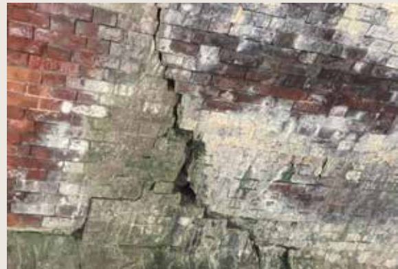
A closeup of structural cracks in the casement.
