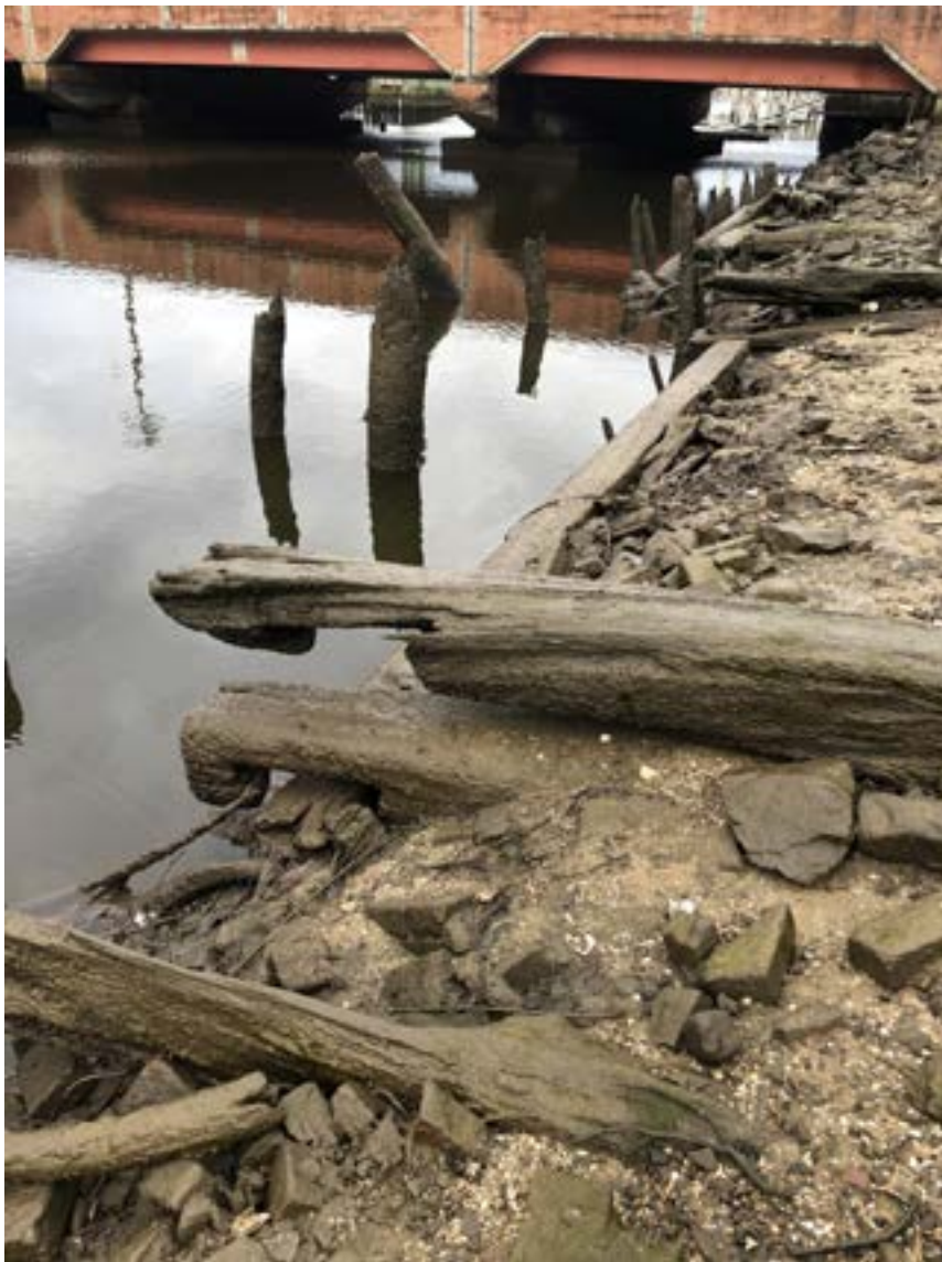
Figure 56. Cribbing west of the Main Street Bridge exposed during an unusually low tide in March 2020.
