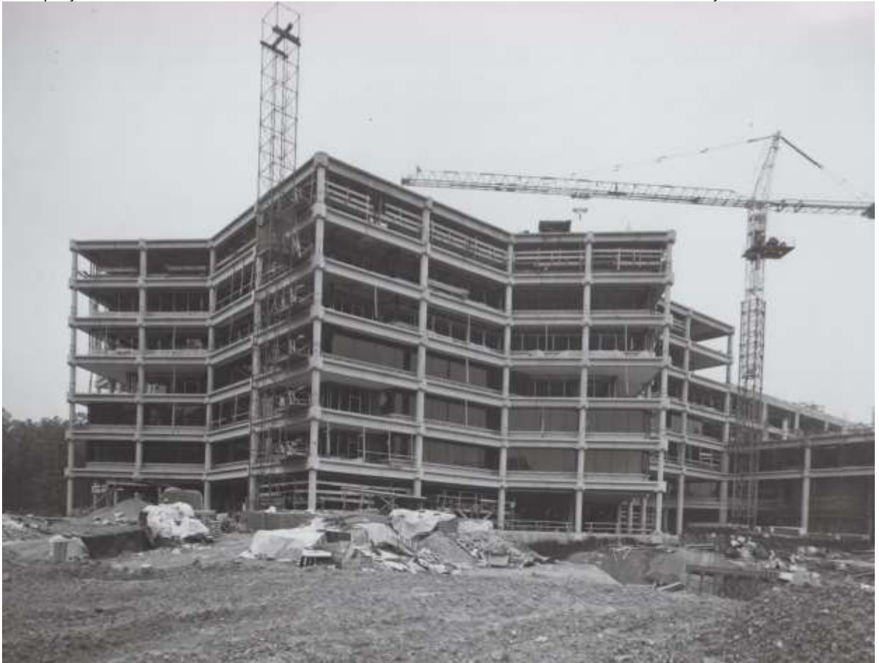
Administration wing of the Powell Federal Building under construction, October 2, 1972 (Clarence King Memorial Library)
