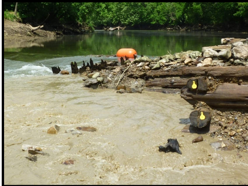
Figure 32: Vertical planks attached to the upstream side of the Section C of the crib dam, and which were removed (May 29, 2019).
