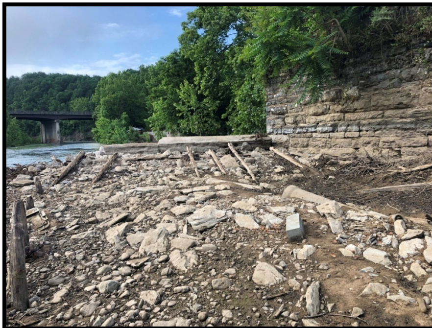
Figure 33: The four angled posts to the left of the abutment are the remnant of the Section A of the crib dam before being covered over. The four vertical members at the bottom left of the photo were removed and are believed to have been “pinning posts” that helped secure the crib dam in place (May 30, 2019).
