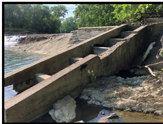
Figure 21: Close-up view of fish ladder, showing deteriorated condition (May 2019).
