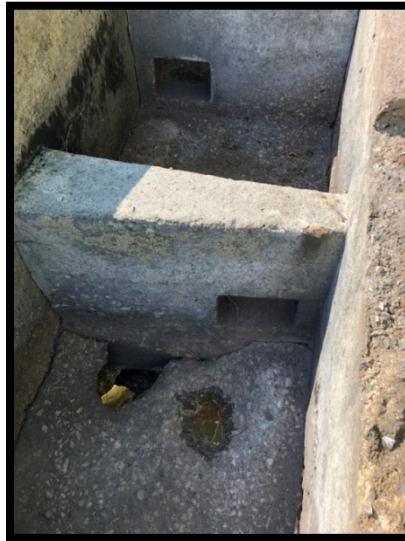
Figure 22: Interior view of the fish ladder showing the pools and the offset orifices in the cross walls to allow for fish passage (May 24).
