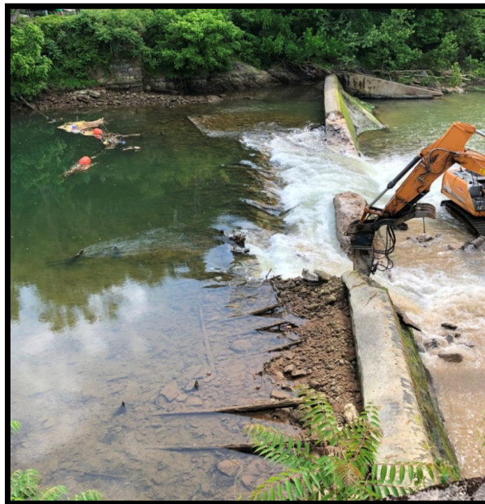
Figure 17: View of dam removal from south abutment on May 24, showing the sloped concrete cap that was applied independently and the makeup of the concrete dam with stones of varying sizes used as aggregate. By this time, the timber crib dam directly upstream was beginning to be exposed.
