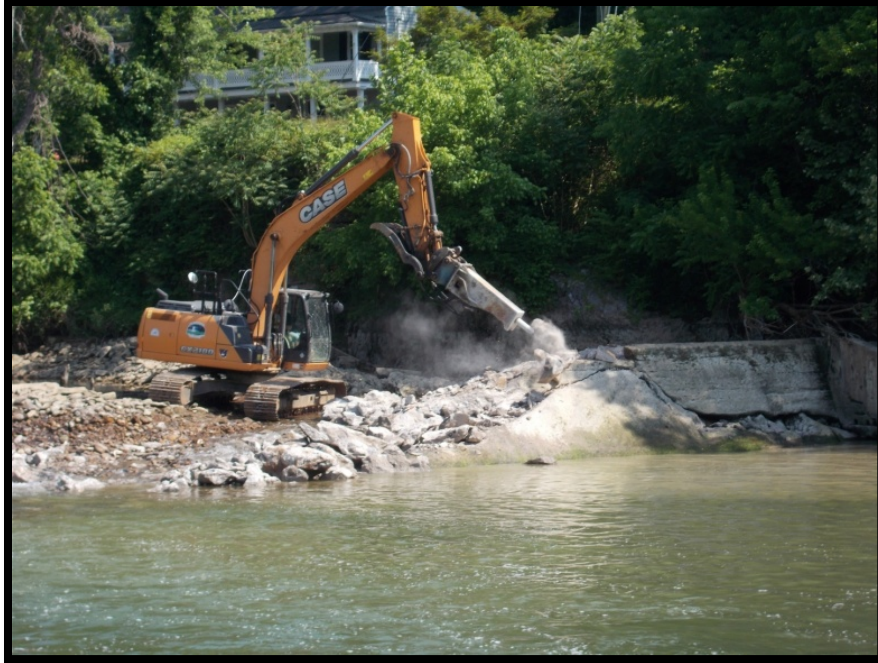
Figure 18: May 25 view of removal of concrete near bedrock and fish ladder at north bank.
