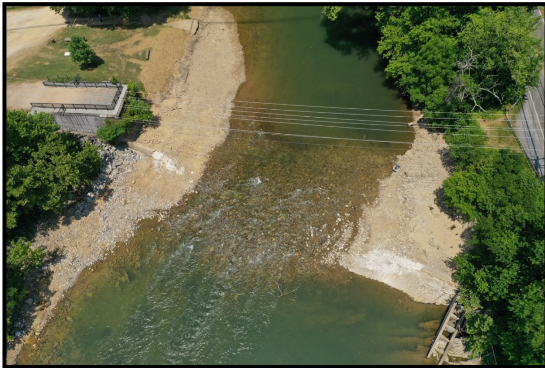
Figure 4: Aerial view showing completed project. Note that parts of the concrete dam on the south side as well as on the north side (along with the fish ladder) remain. The portion of the crib dam at the southern abutment has been covered as has some of the structural remnant. (David Pfaff, W&L University)
