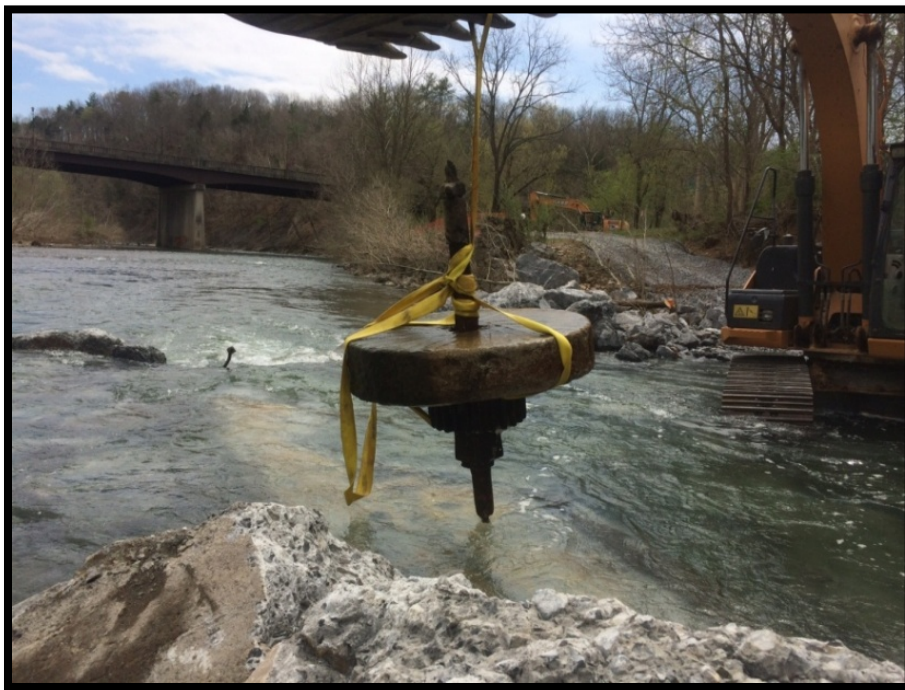
Figure 38: Removal of millstone from Maury River on April 11, 2019.
