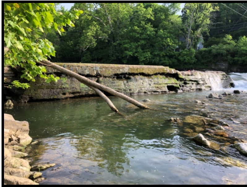
Figure 16: View from downstream south end, showing poor condition of dam wall and distinct joint between wall of dam and the cap (May 24).
