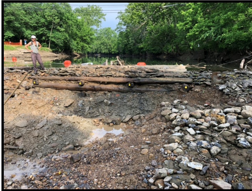
Figure 30: East side of Section D crib that was numbered and salvaged (May 29, 2019).
